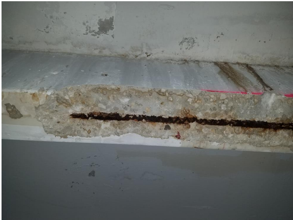
Photo 8: Joist Reinforcement was severely corroded
