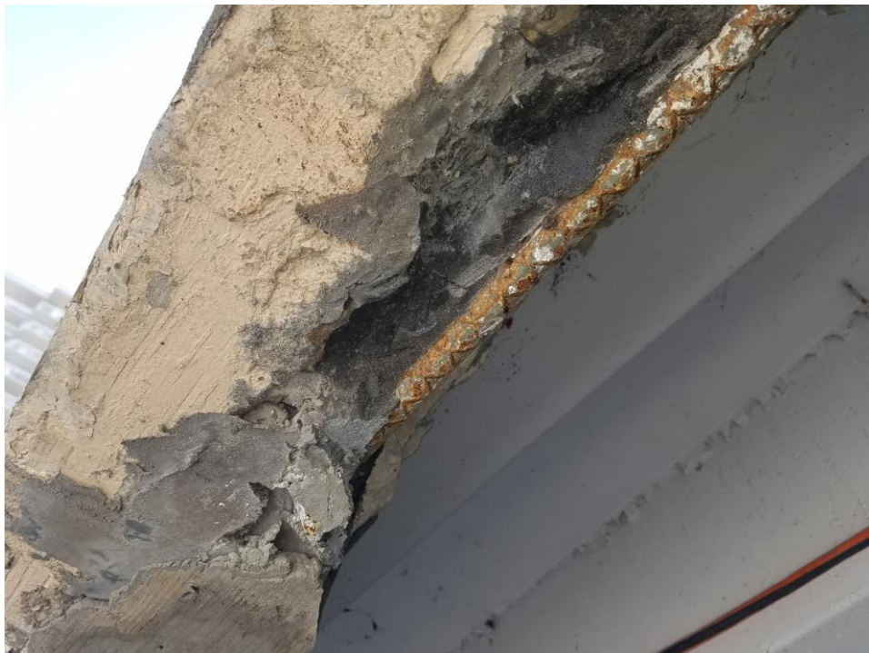
Photo 16: Evidence of minor corrosion in the reinforcement and poorly repaired concrete beam
