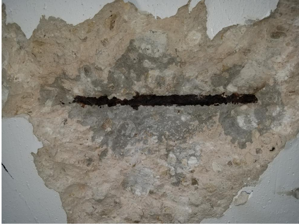
Photo 3: Reinforcement was not cleaned, and corrosion was present
