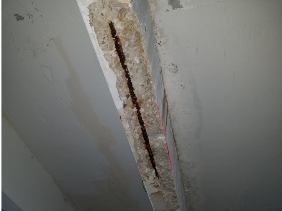
Photo 7: No concrete repairs were performed at the joint
