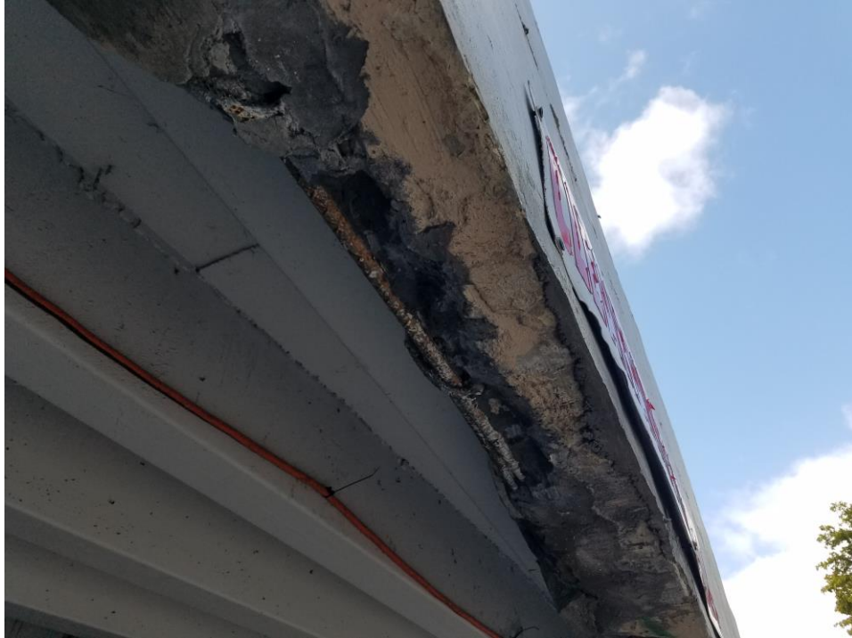
Photo 15: Sub-standard concrete repair. Evidence of minor corrosion in the reinforcement
