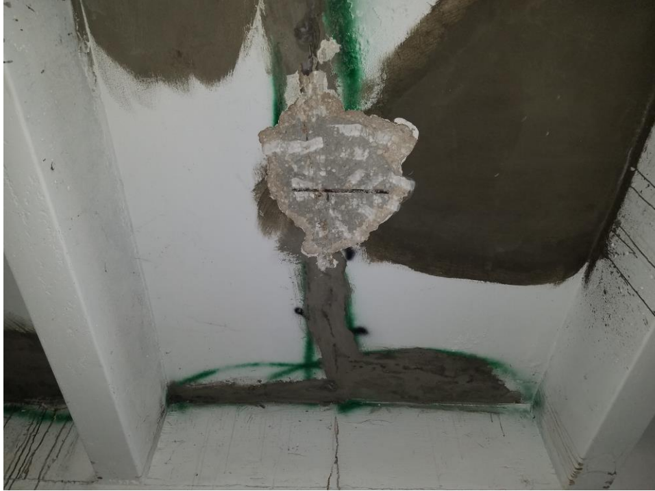
Photo 5: Minor corrosion was observed at the reinforcement
