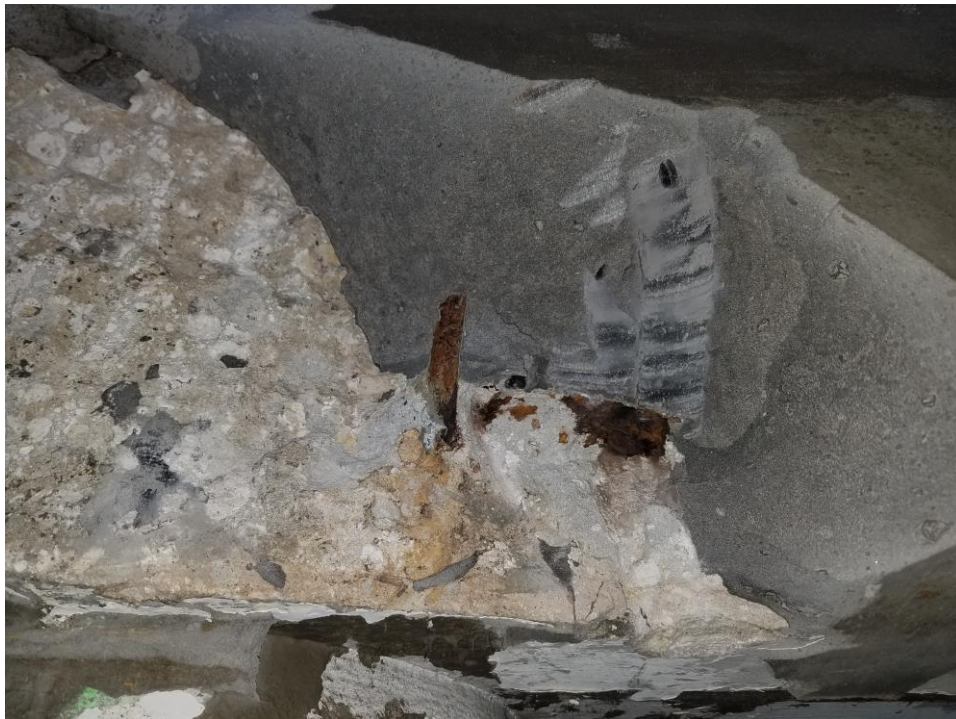
Photo 12: Evidence of corrosion in the reinforcement.
