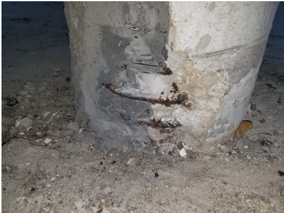
Photo 10: Evidence of corrosion in the column reinforcement
