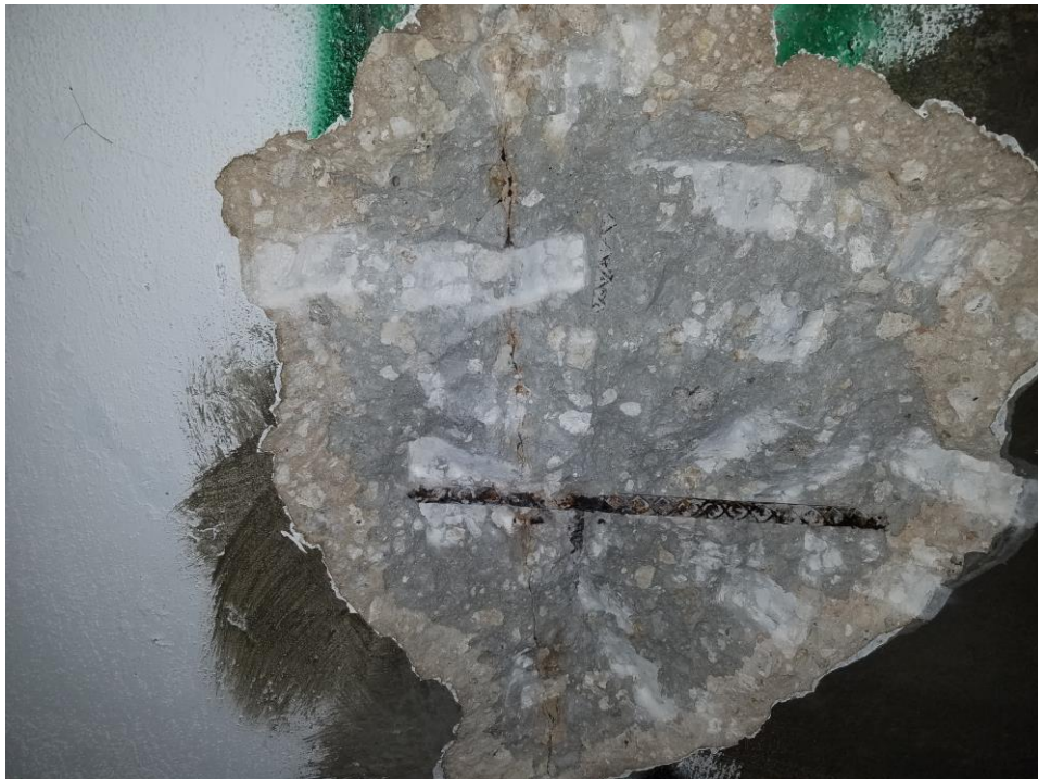
Photo 6: Epoxy was not present at the Crack in overhead slab
