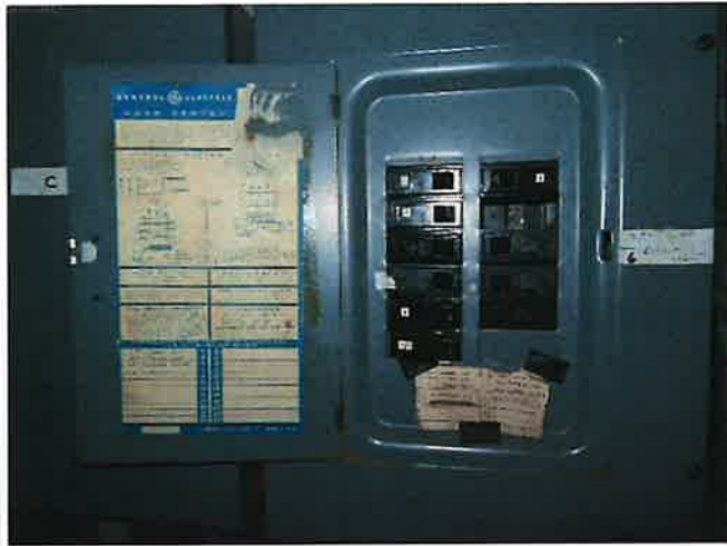
Photo # 49. North building - electrical panel depicted (item #4.35)
