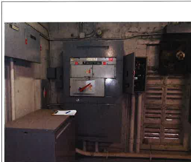
Photo # 3. Unidentified service-disconnect switch (main electrical room South building)
