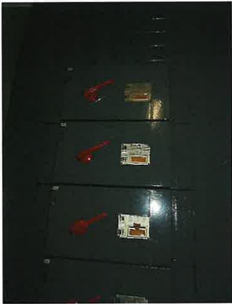
Photo # 21. North building main electrical room electrical panel depicted (item #4.7)
