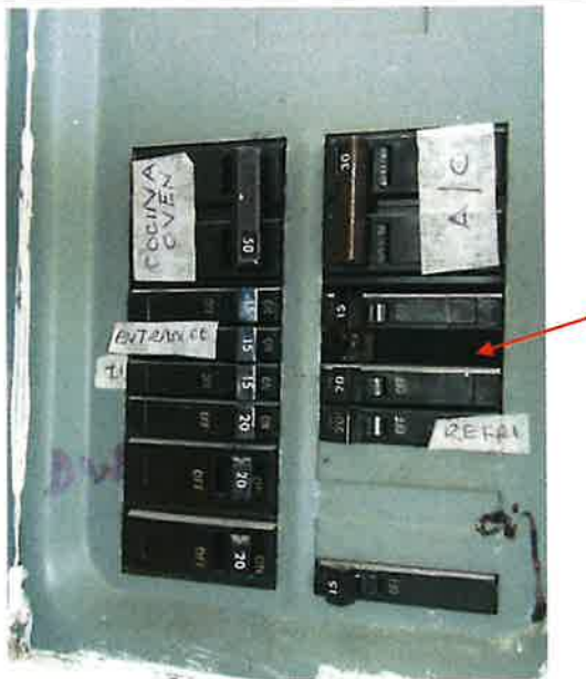
Photo # 91. Typical residential panel having an opening in a circuit space (item #4.71)
