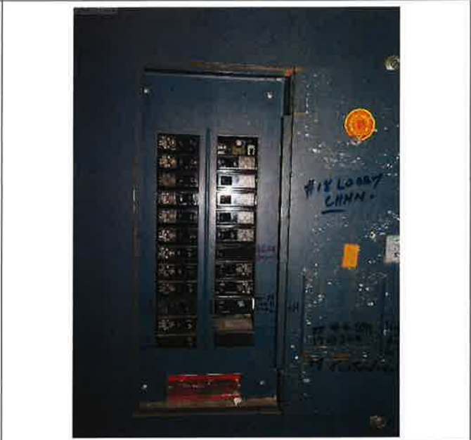
Photo # 82. South building - electrical panel depicted (item #4.65)
