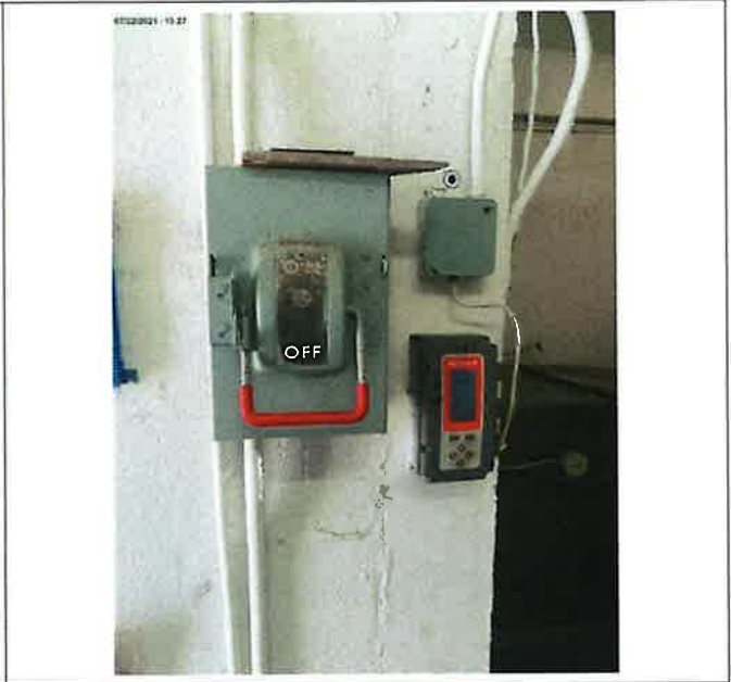
Photo # 114. Disconnect switch not labeled to identify the load it serves (South building, roof cooling tower mechanical room)(Item #10.a.3)
