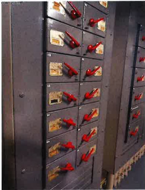
Photo # 19. North building main electrical room electrical panel depicted (item #4.5)
