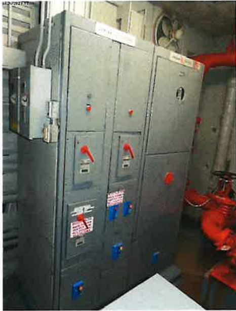
Photo # 1. Unidentified service-disconnect switch (main electrical room North building)
