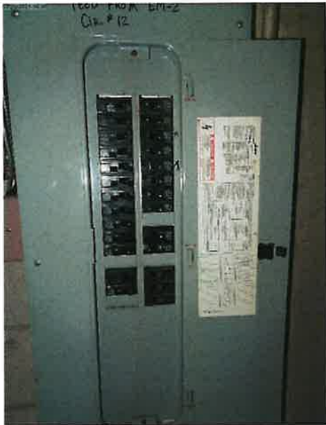
Photo # 81. South building - electrical panel depicted (item #4.64)
