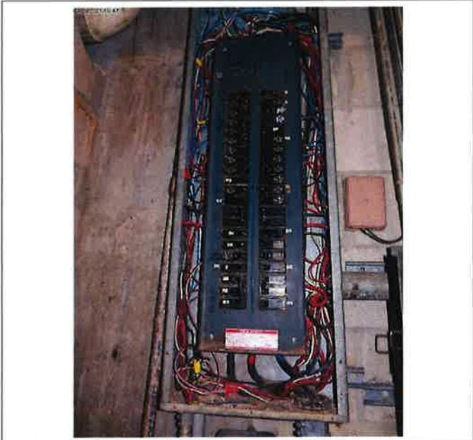
Photo # 83. South building - electrical panel depicted (item #4.66)
