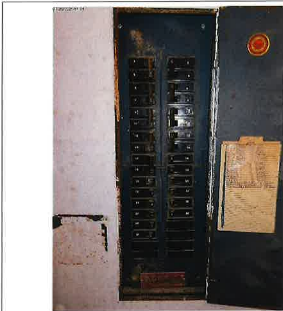
Photo # 69. South building - electrical panel depicted (item #4.54)
