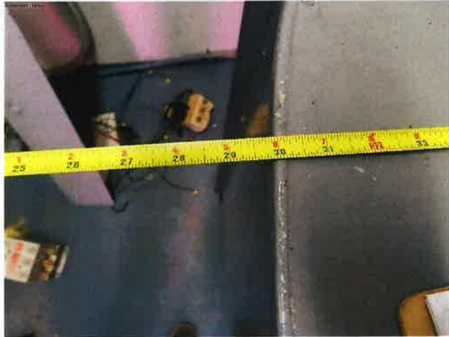
Photo # 125. Working space clearance violation (Item # 10-SOUTH-h)
