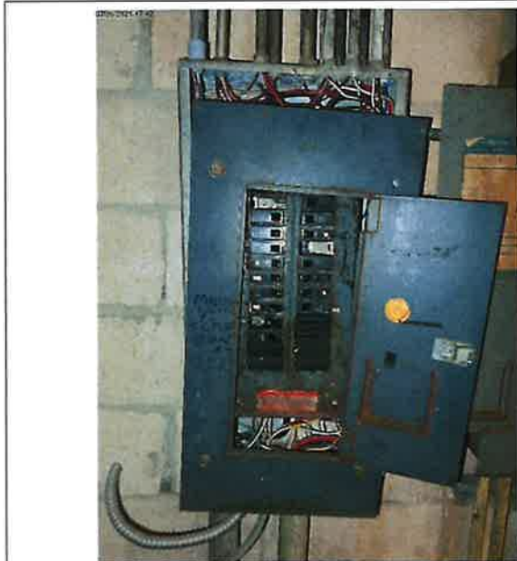
Photo # 43. North building - electrical panel depicted (item #4.29)
