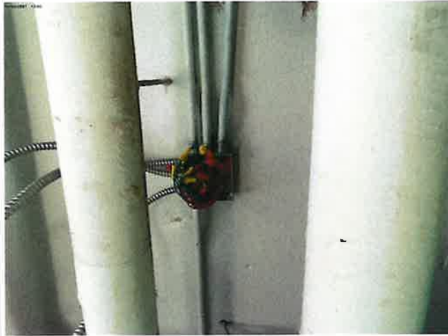
Photo # 109. Opening in junction boxes/enclosures (Item #10.f.2)
