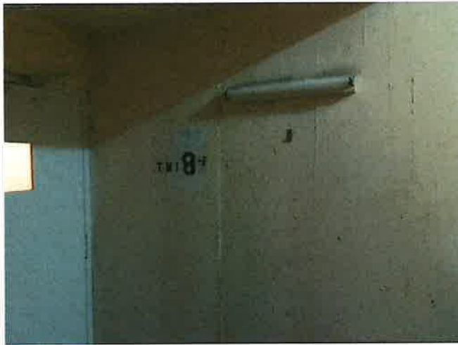
Photo # 133. Insufficient illumination for the building means of egress (Item #13.NORTH-e).
