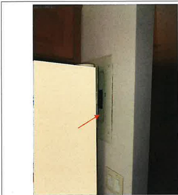
Photo # 93. Typical residential panel where there is no working space clearance (item #4.71)
