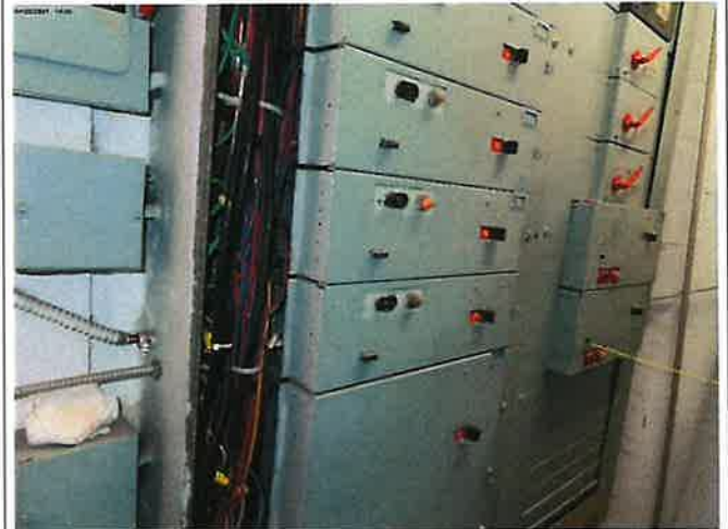
Photo # 128. Missing protective cover for the motor control center (Item # 10-SOUTH-i)
