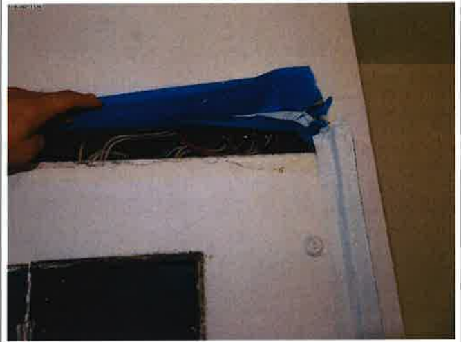
Photo # 74. South building - electrical panel depicted (item #4.59)
