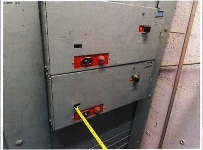
Photo # 126. Working space clearance violation (Item # 10-SOUTH-h)
