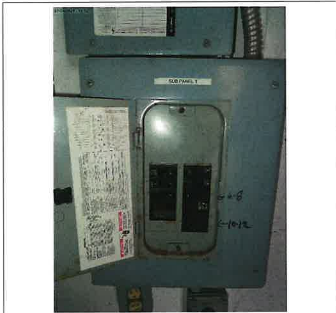
Photo # 29. North building - electrical panel depicted (item #4.15)
