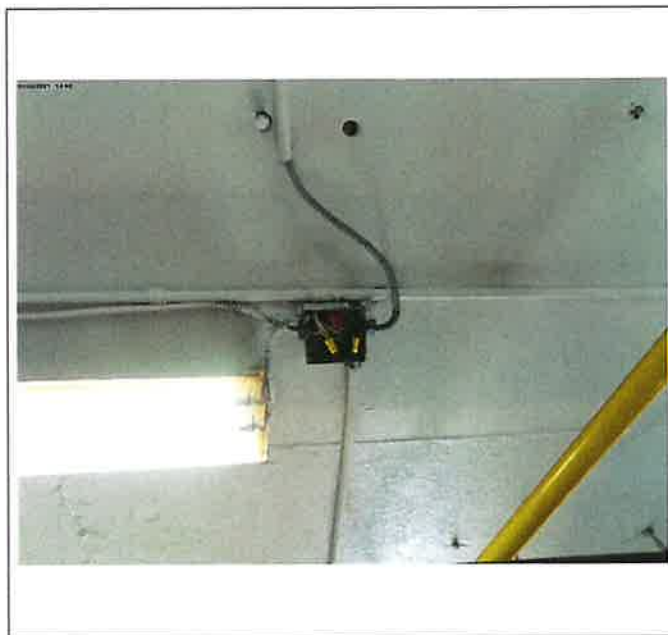
Photo # 107. Opening in junction boxes/enclosures (Item #10.f.2)
