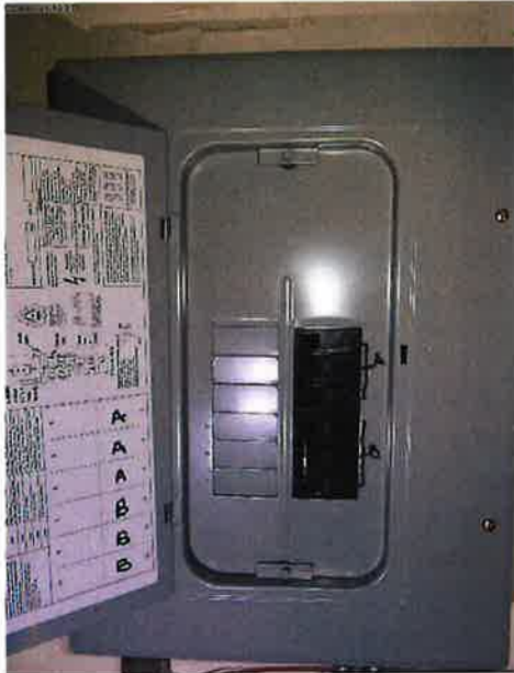
Photo # 45. North building - electrical panel depicted (item #4.31)
