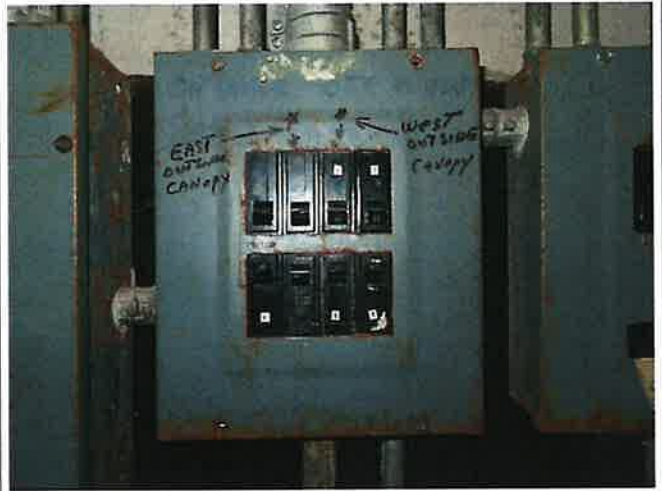
Photo # 42. North building - electrical panel depicted (item #4.28)
