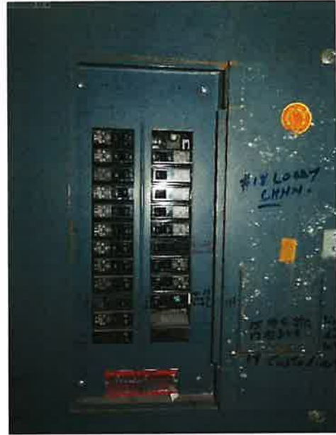
Photo # 82. South building - electrical panel depicted (item #4.65)
