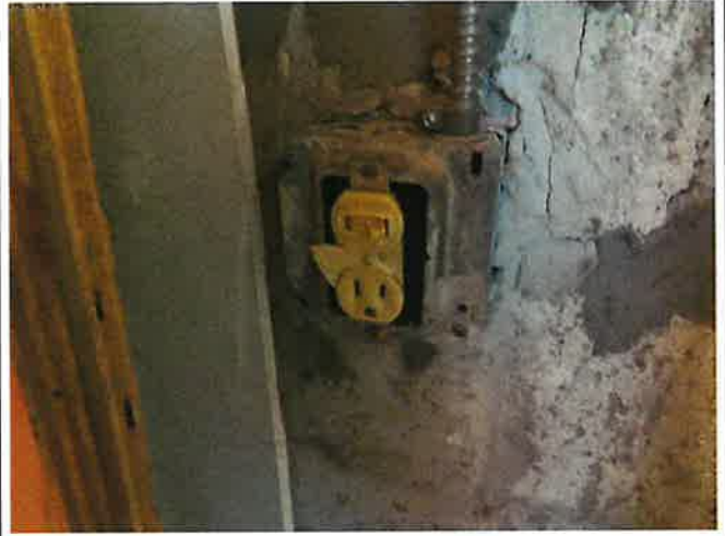
Photo # 102. North building, tower 3, PH level storage room: receptacle missing protective cover.
