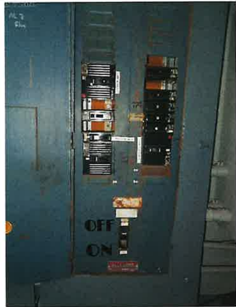
Photo # 18. North building main electrical room electrical panel depicted (item #4.4)
