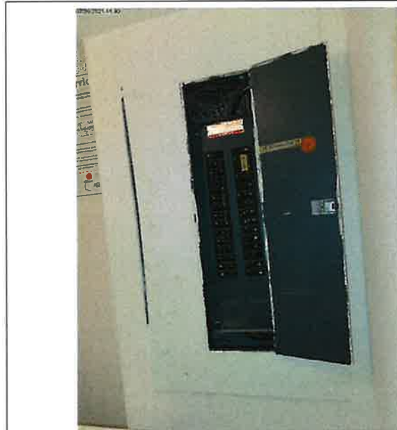
Photo # 67. South building - electrical panel depicted (item #4.52)
