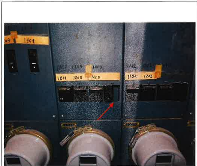
Photo # 9. North building, tower 4, meter room level 12: opening in circuit breaker space.
