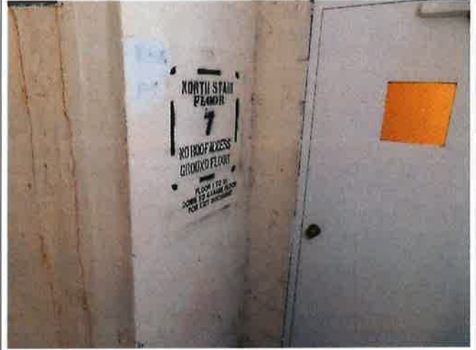
Photo # 134. Insufficient illumination for the building means of egress (Item #13.NORTH-f).
