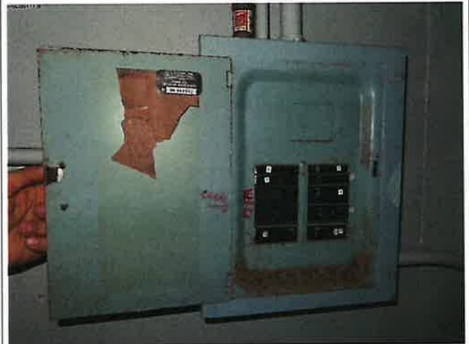
Photo # 24. North building main electrical room electrical panel depicted (item #4.10)
