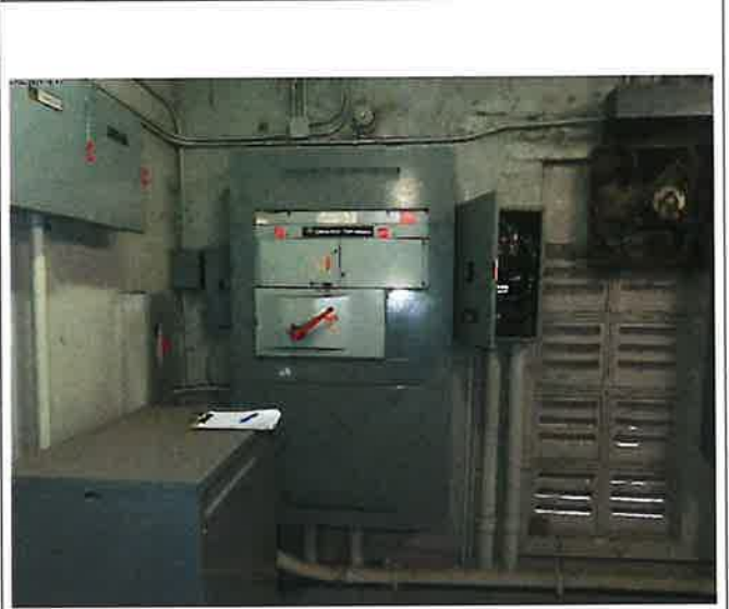
Photo # 54. South building main electrical room electrical panel depicted (item #4.39)
