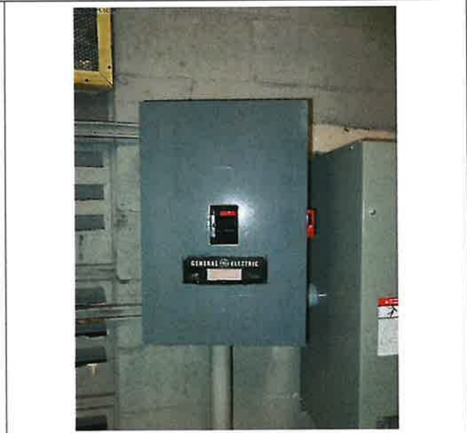
Photo # 116. Disconnect switch not labeled to identify the load it serves (South building, roof cooling tower mechanical room)(Item #10.a.5)
