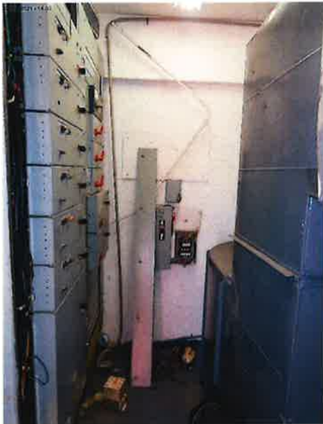
Photo # 127. Working space clearance violation (Item # 10-SOUTH-h)
