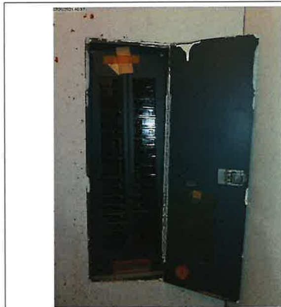
Photo # 35. North building - electrical panel depicted (item #4.21)
