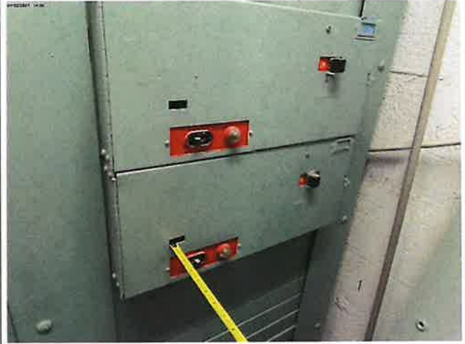
Photo # 126. Working space clearance violation (Item # 10-SOUTH-h)
