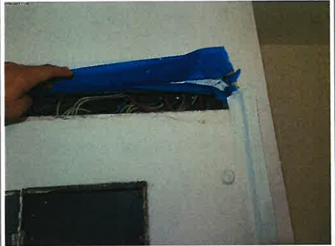
Photo # 74. South building - electrical panel depicted (item #4.59)
