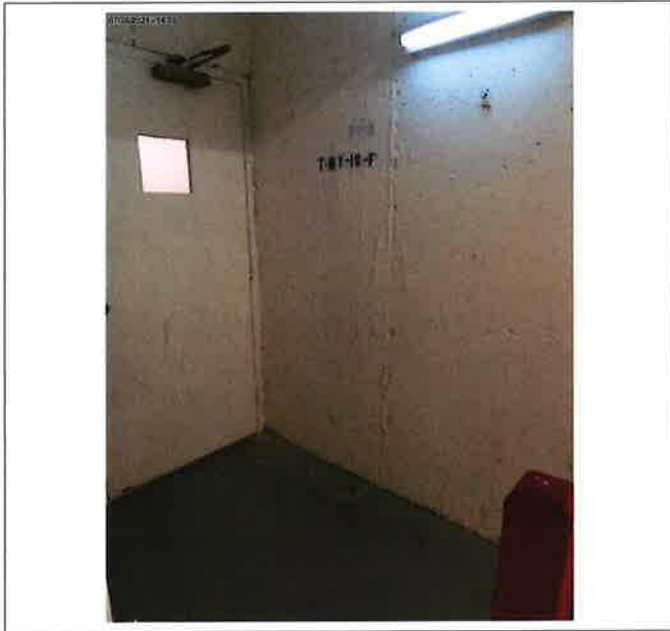
Photo # 131. Insufficient illumination for the building means of egress (Item #13.NORTH-c).
