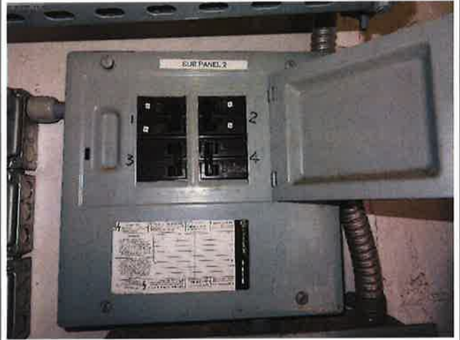
Photo # 30. North building - electrical panel depicted (item #4.16)
