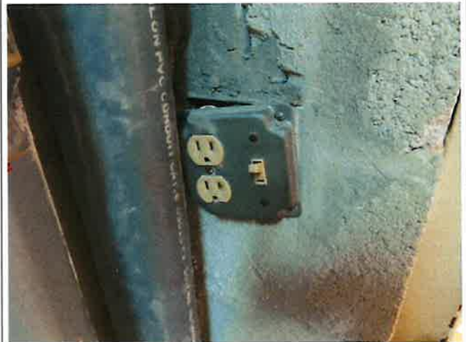
Photo # 120. Receptacle and switch not properly secured to the box (Item # 10-SOUTH-d)
