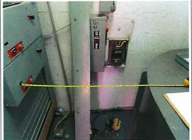
Photo # 124. Working space clearance violation (Item # 10-SOUTH-h)
