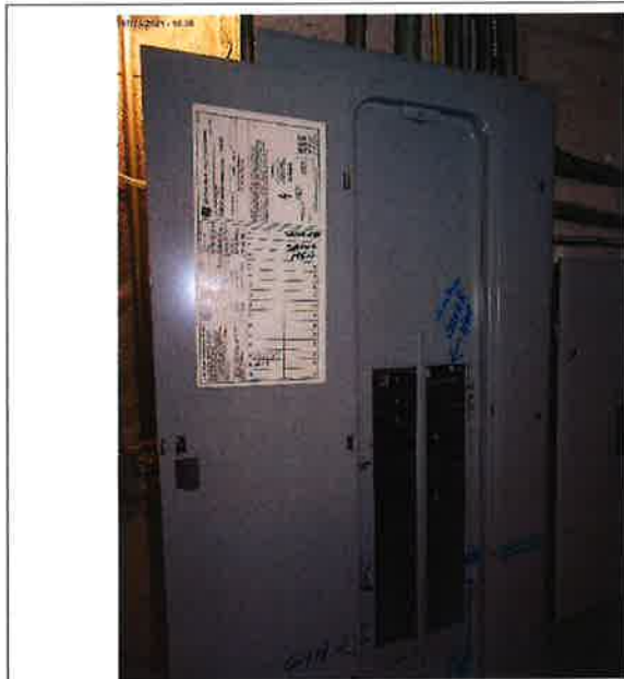
Photo # 39. North building - electrical panel depicted (item #4.25)
