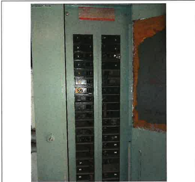
Photo # 61. South building - electrical panel depicted (item #4.48)
