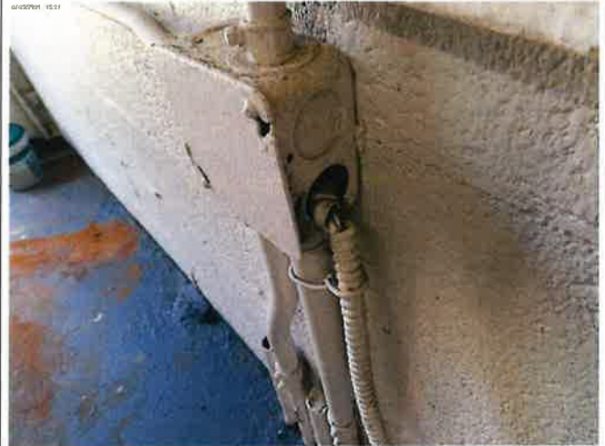
Photo # 118. Conduit mechanically detached (Item # 10-SOUTH-c)
