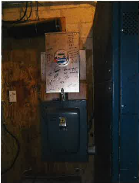
Photo # 117. Disconnect switch not labeled to identify the load it serves (South building, roof cooling tower mechanical room)(Item #10.a.6)
