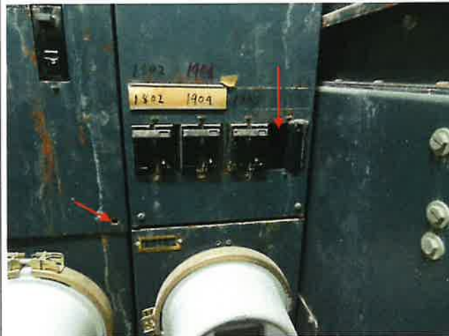
Photo # 7. North building, tower 3, meter room level 19: opening in meter can. Notice the circuit breaker cover is missing screws.
