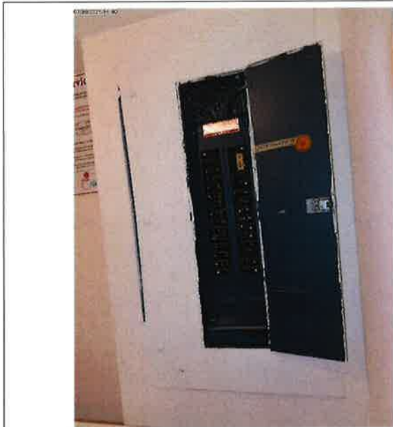
Photo # 67. South building - electrical panel depicted (item #4.52)
