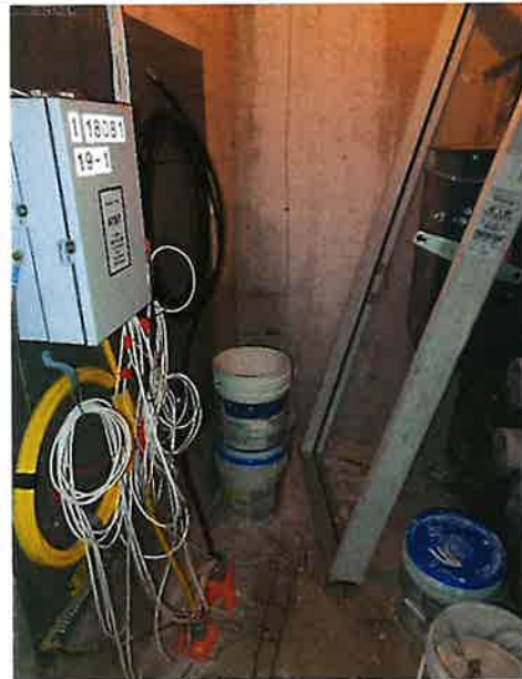
Photo # 4. Meter rooms were found use for storage purposes
