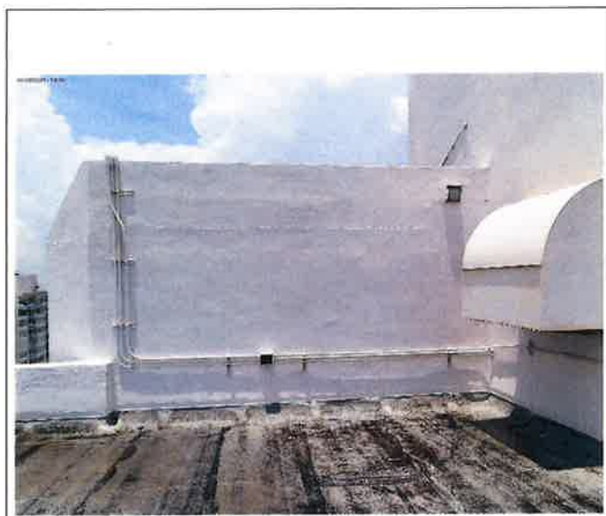
Photo # 105. Opening in junction boxes/enclosures (Item #10.f.1)
