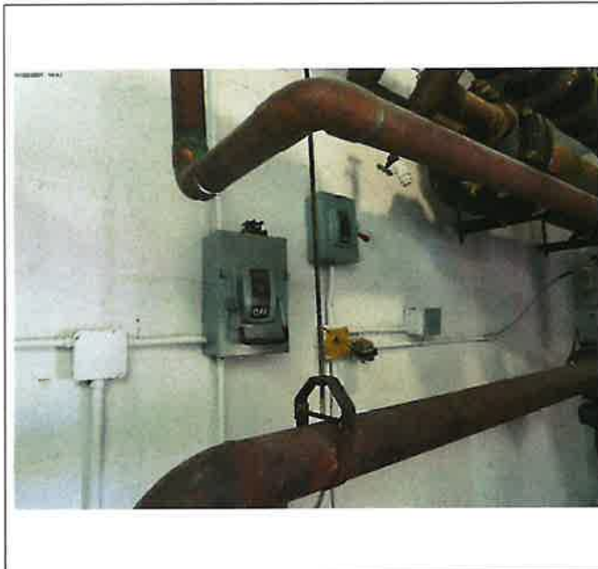
Photo # 113. Disconnect switch not labeled to identify the load it serves (South building, roof cooling tower mechanical room)(Item #10.a.2)
