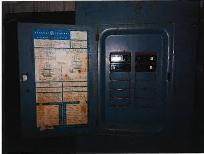
Photo # 41. North building - electrical panel depicted (item #4.27)
