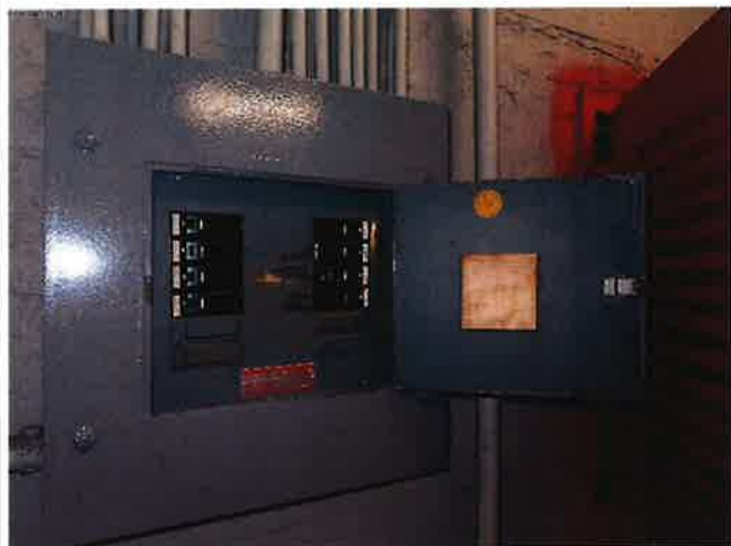
Photo # 59. South building main electrical room electrical panel depicted (item #4.44)
