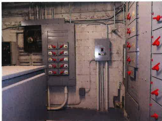
Photo # 55. South building main electrical room electrical panel depicted (item #4.40)
