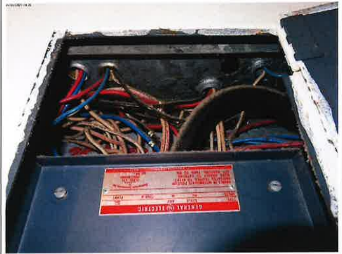
Photo # 66. South building - electrical panel depicted (item #4.52)
