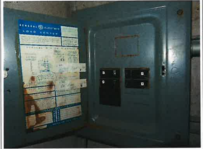
Photo # 78. South building - electrical panel depicted (item #4.61)
