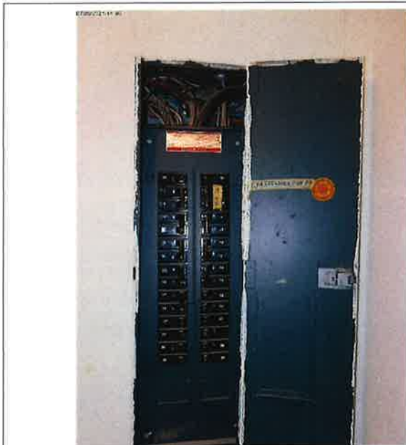
Photo # 65. South building - electrical panel depicted (item #4.52)
