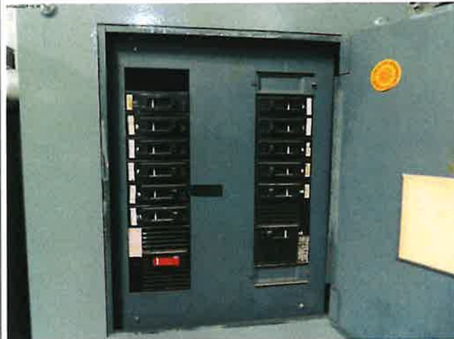
Photo # 51. South building main electrical room electrical panel depicted (item #4.37)
