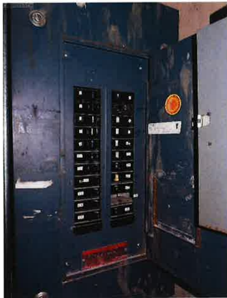
Photo # 47. North building - electrical panel depicted (item #4.33)
