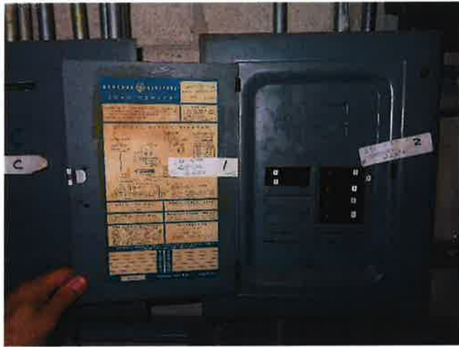
Photo # 85. South building - electrical panel depicted (item #4.68)
