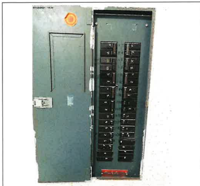
Photo # 31. North building - electrical panel depicted (item #4.17)
