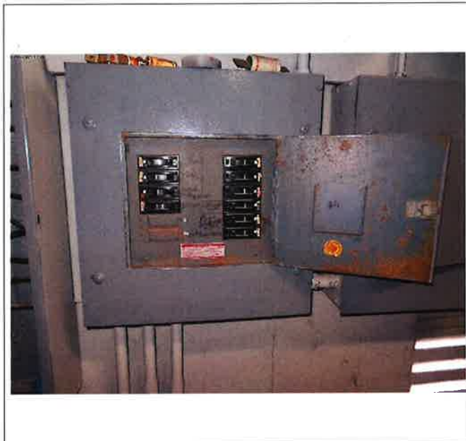
Photo # 15. North building main electrical room electrical panel depicted (item #4.2)
