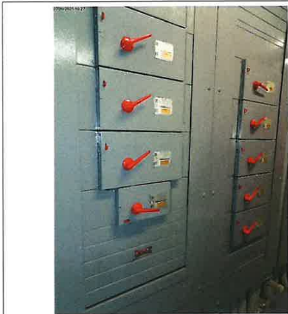
Photo # 57. South building main electrical room electrical panel depicted (item #4.42)
