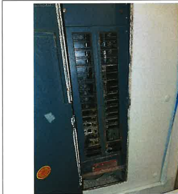
Photo # 75. South building - electrical panel depicted (item #4.59)
