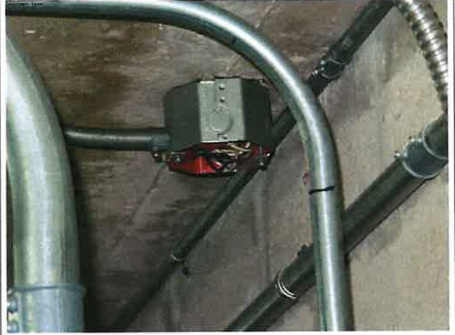
Photo # 110. Opening in junction boxes/enclosures (Item #10.f.3)
