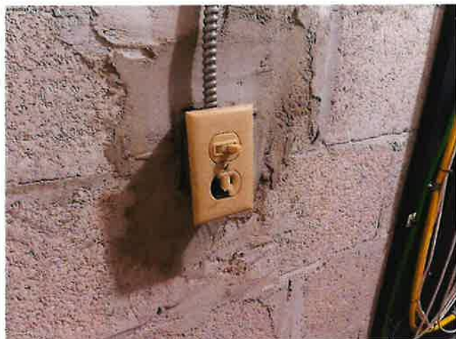
Photo # 103. Broken receptacle cover, meter room level 16, North building, tower 2.
