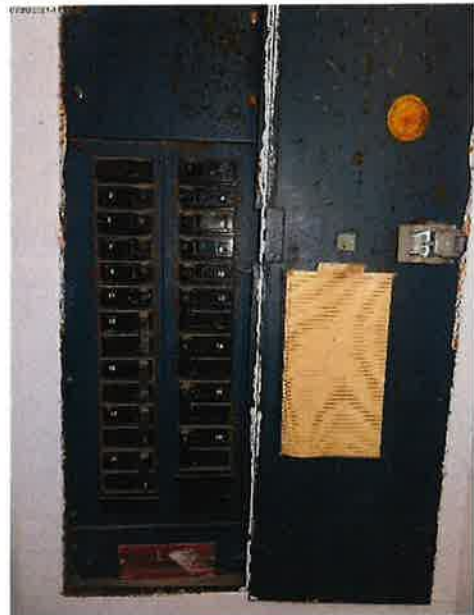
Photo # 38. North building - electrical panel depicted (item #4.24)
