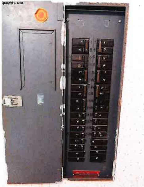
Photo # 31. North building - electrical panel depicted (item #4.17)
