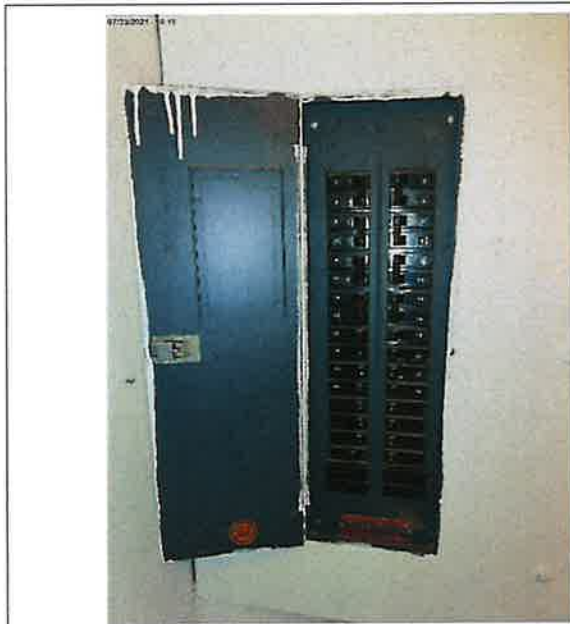
Photo # 33. North building - electrical panel depicted (item #4.19)
