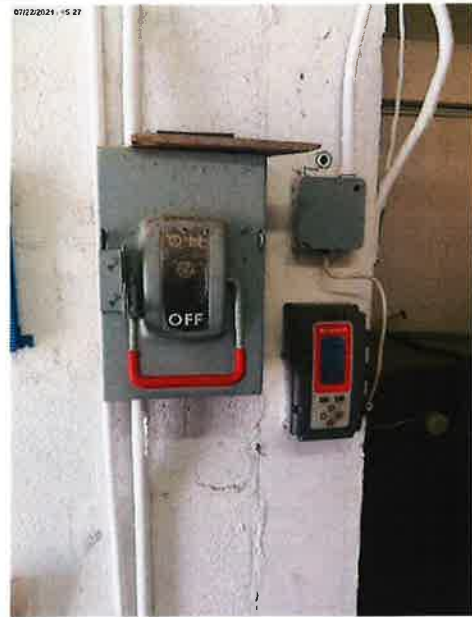
Photo # 114. Disconnect switch not labeled to identify the load it serves (South building, roof cooling tower mechanical room)(Item #10.a.3)
