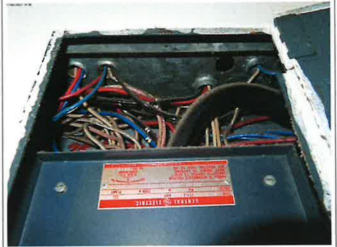
Photo # 66. South building - electrical panel depicted (item #4.52)
