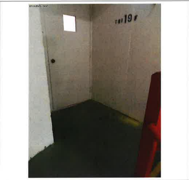
Photo # 130. Insufficient illumination for the building means of egress (Item #13.NORTH-b).
