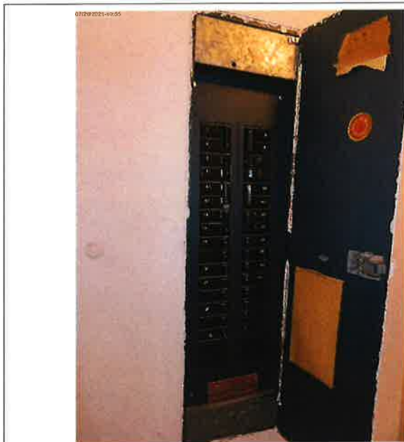
Photo # 37. North building - electrical panel depicted (item #4.23)
