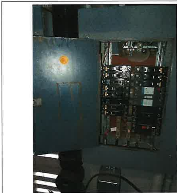
Photo # 17. North building main electrical room electrical panel depicted (item #4.3)
