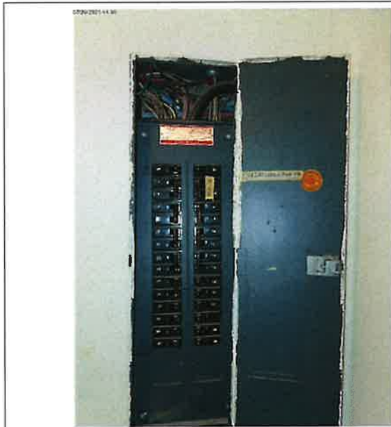
Photo # 65. South building - electrical panel depicted (item #4.52)
