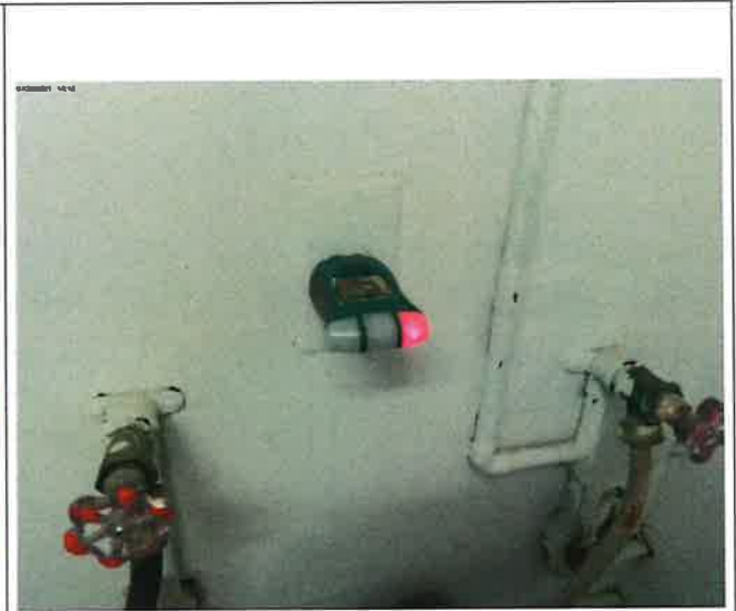
Photo # 96. Laundry room receptacle for the washer machine is depicted. Notice the grounding is missing. Also, GFCI protection is required (typical for all level, all towers in both buildings)
