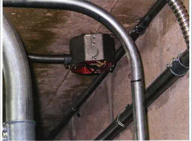
Photo # 110. Opening in junction boxes/enclosures (Item #10.f.3)
