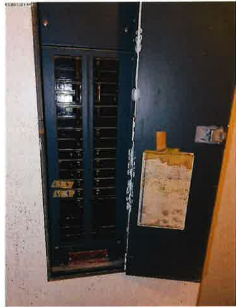
Photo # 70. South building - electrical panel depicted (item #4.55)
