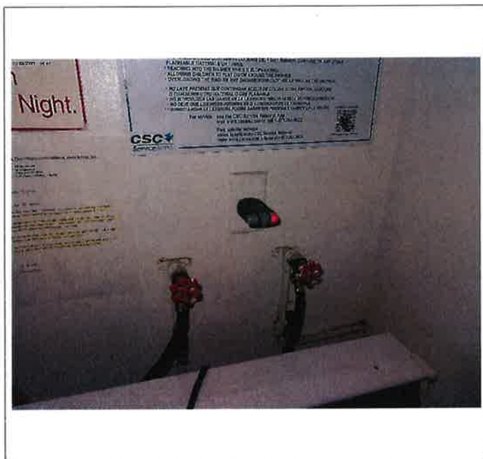
Photo # 99. Laundry room receptacle for the washer machine is depicted. Notice the grounding is missing. Also, GFCI protection is required (typical for all level, all towers in both buildings) (Item #10.b)
