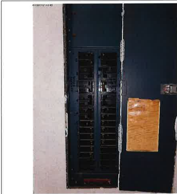
Photo # 71. South building - electrical panel depicted (item #4.57)
