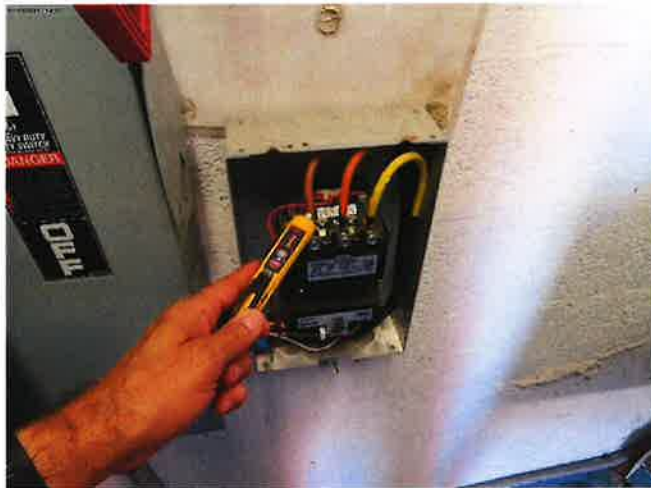
Photo # 123. Opening in junction box exposing live wires (Item # 10-SOUTH-g.2)
