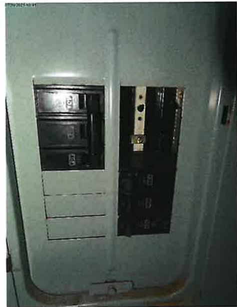
Photo # 50. North building - electrical panel depicted (item #4.36)
