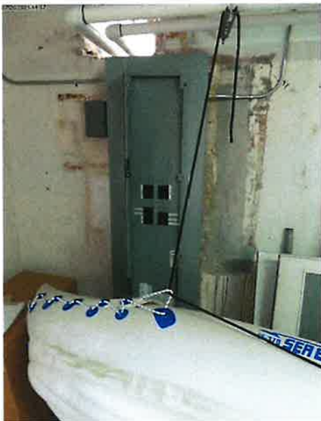
Photo # 87. Marina storage room (under the pool deck) – electrical panel depicted (item #4.70)
