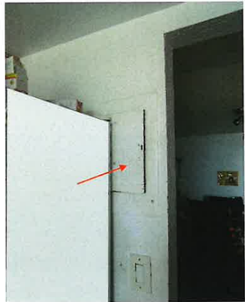
Photo # 94. Typical residential panel where there is no working space clearance (item #4.71)
