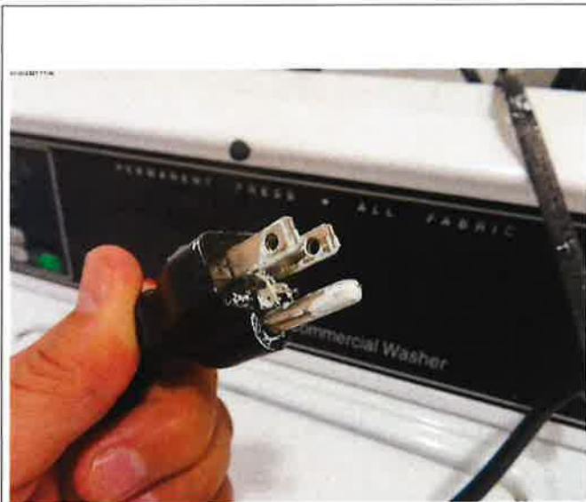
Photo # 101. A plug for the washer machine is depicted. Notice paint covering the metal connectors which impeach proper grounding. Plug connectors must be cleaned (typical) (Item #10.b)
