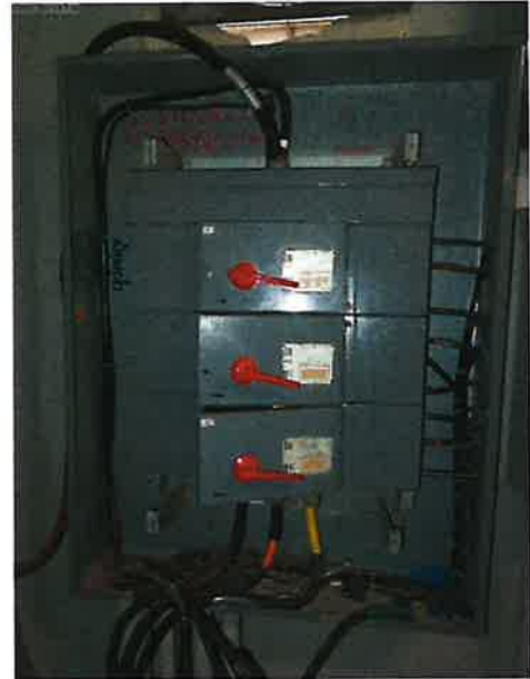
Photo # 14. North building main electrical room electrical panel depicted (item #4.1)
