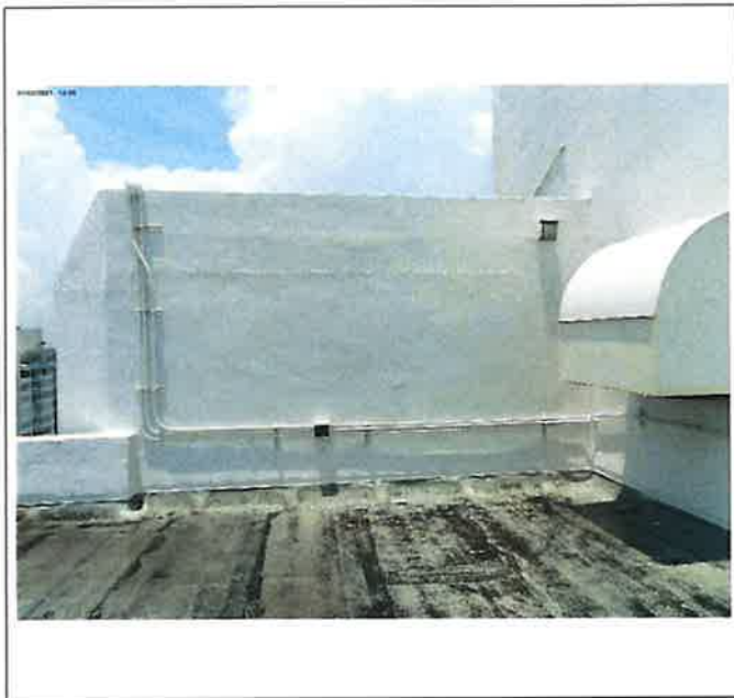
Photo # 105. Opening in junction boxes/enclosures (Item #10.f.1)
