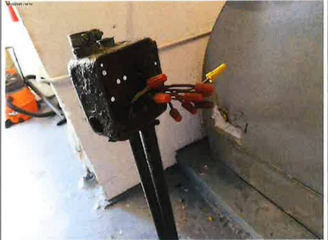
Photo # 122. Opening in junction box exposing live wires (Item # 10-SOUTH-g.1)
