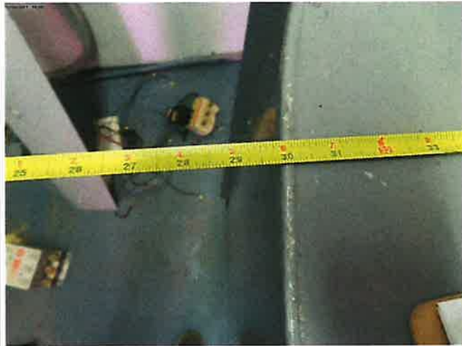
Photo # 125. Working space clearance violation (Item # 10-SOUTH-h)
