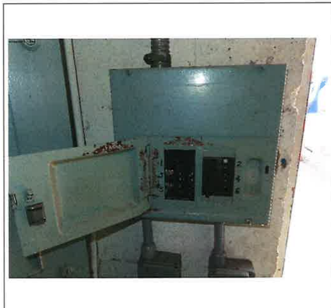
Photo # 63. South building - electrical panel depicted (item #4.50)
