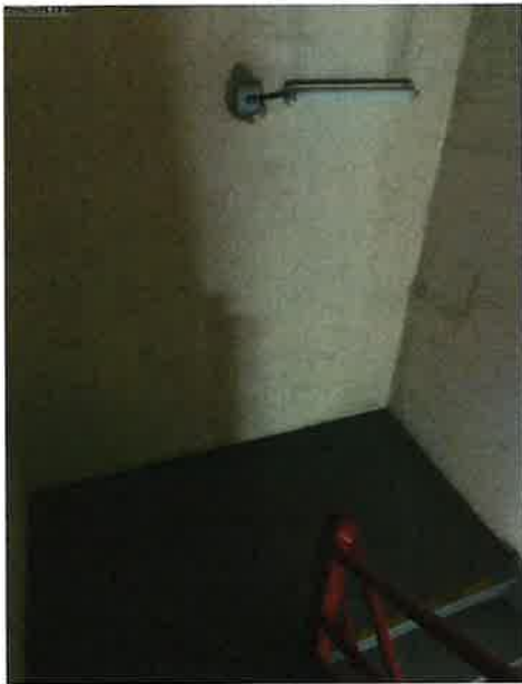
Photo # 139. Insufficient illumination for the building means of egress (Item #13.SOUTH-c).
