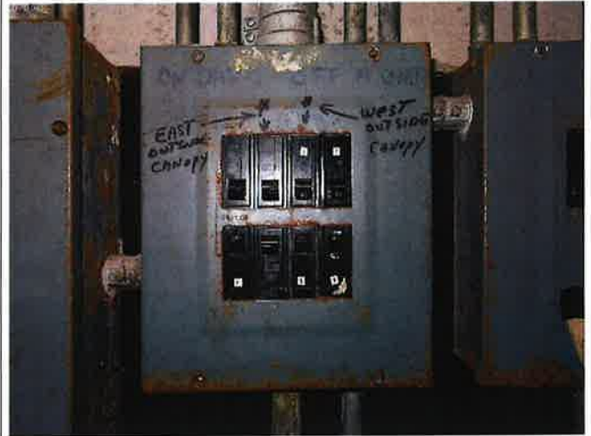
Photo # 42. North building - electrical panel depicted (item #4.28)
