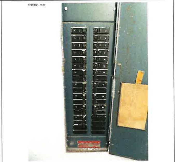
Photo # 34. North building - electrical panel depicted (item #4.20)
