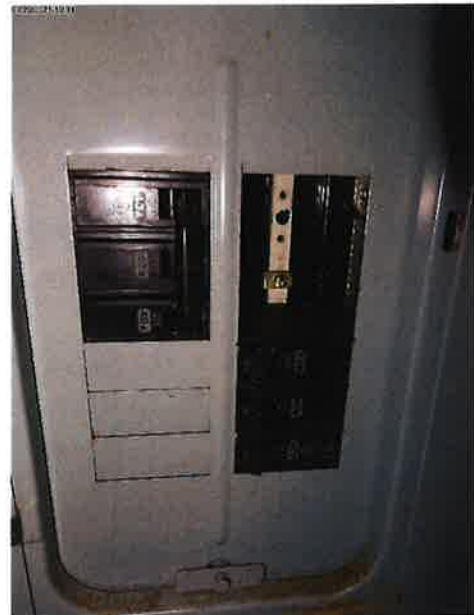
Photo # 50. North building - electrical panel depicted (item #4.36)
