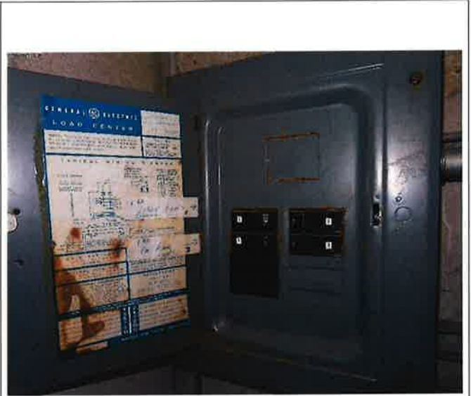
Photo # 78. South building - electrical panel depicted (item #4.61)
