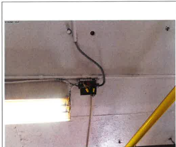
Photo # 107. Opening in junction boxes/enclosures (Item #10.f.2)
