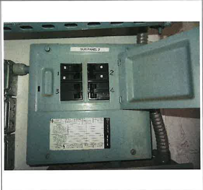
Photo # 30. North building - electrical panel depicted (item #4.16)
