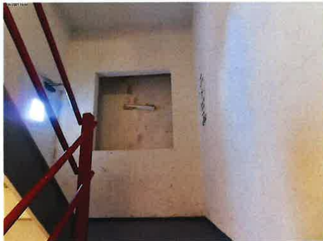
Photo # 135. Insufficient illumination for the building means of egress (Item #13.SOUTH-a).
