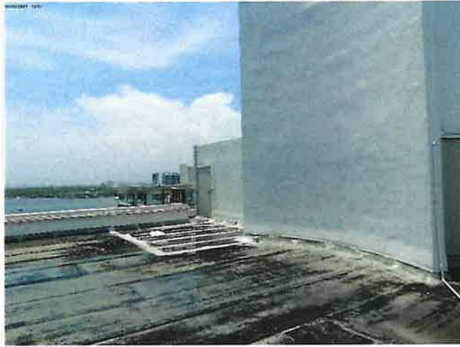
Photo # 141. North building roof: Stairwell exit doors are missing exit sign (Item # 16.a)
