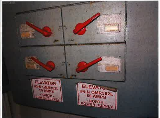
Photo # 26. North building - electrical panel depicted (item #4.12)
