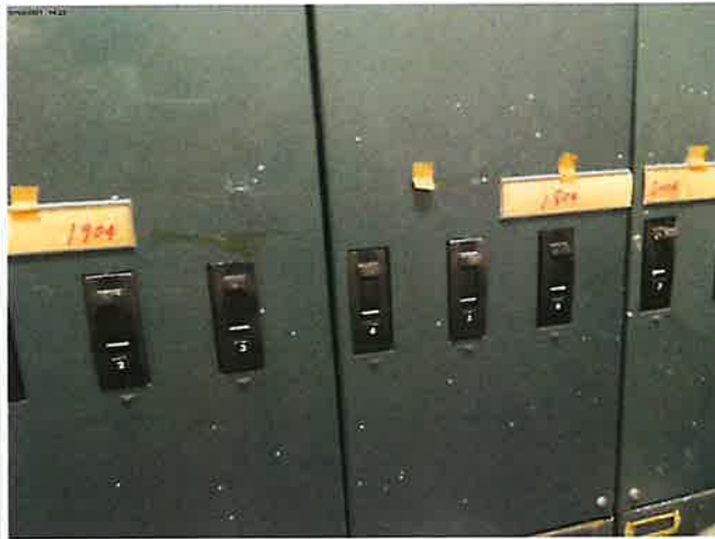
Photo # 5. Some main circuit breakers in the meter cans are missing identification of the unit they serve.
