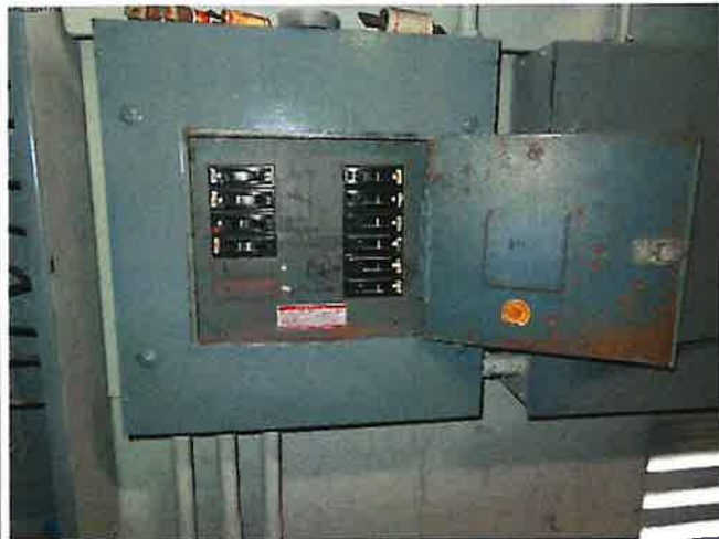
Photo # 15. North building main electrical room electrical panel depicted (item #4.2)
