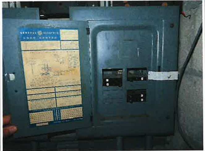
Photo # 86. South building - electrical panel depicted (item #4.69)
