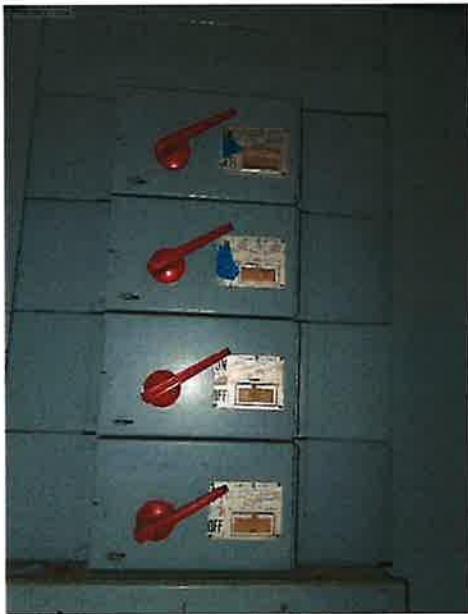
Photo # 27. North building - electrical panel depicted (item #4.13)
