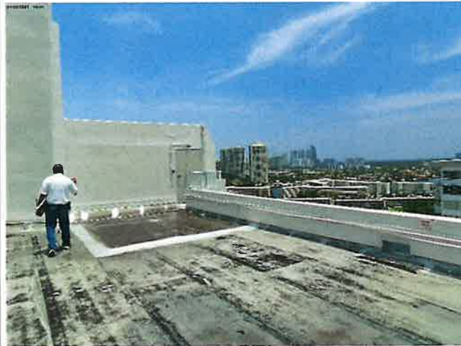
Photo # 143. North building roof: Stairwell exit doors are missing exit sign (Item # 16.a)
