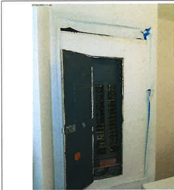
Photo # 73. South building - electrical panel depicted (item #4.59)
