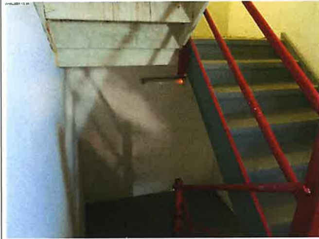
Photo # 137. Insufficient illumination for the building means of egress (Item #13.SOUTH-b).
