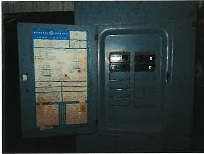
Photo # 41. North building - electrical panel depicted (item #4.27)
