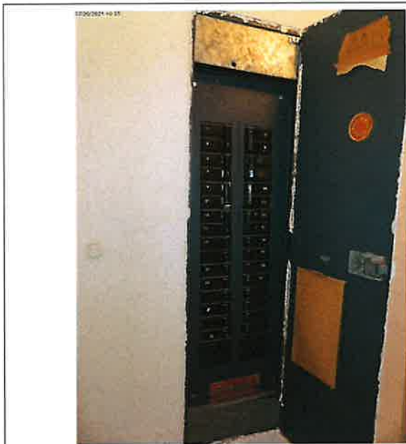
Photo # 37. North building - electrical panel depicted (item #4.23)
