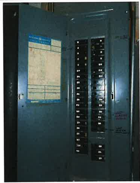
Photo # 46. North building - electrical panel depicted (item #4.32)
