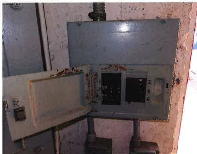
Photo # 63. South building - electrical panel depicted (item #4.50)
