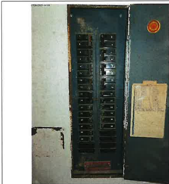
Photo # 69. South building - electrical panel depicted (item #4.54)
