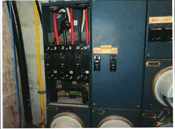
Photo # 6. North building tower 1, meter bank level 3: missing cover for meter can circuit breaker enclosure.
