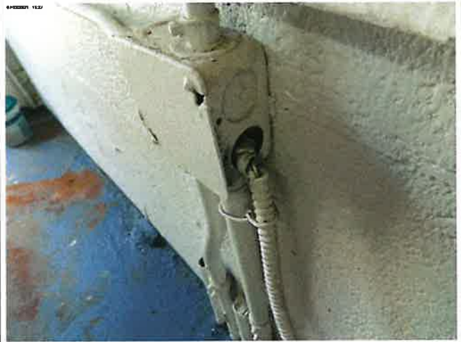
Photo # 118. Conduit mechanically detached (Item # 10-SOUTH-c)
