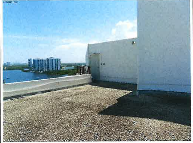
Photo # 146. South building roof: Stairwell exit doors are missing exit sign (Item # 16.b)
