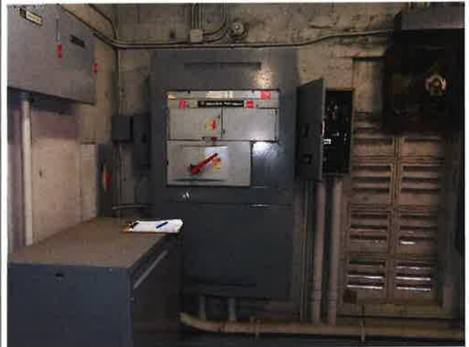
Photo # 54. South building main electrical room electrical panel depicted (item #4.39)
