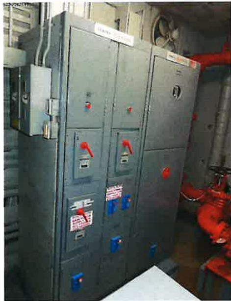
Photo # 23. North building main electrical room electrical panel depicted (item #4.9)
