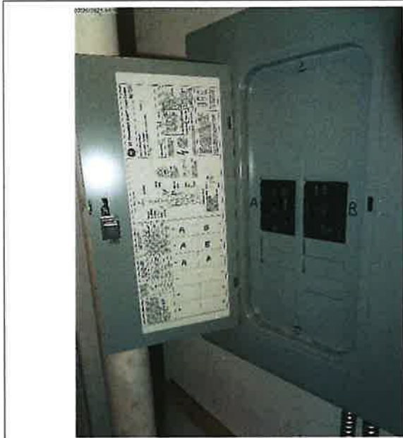
Photo # 77. South building - electrical panel depicted (item #4.60)
