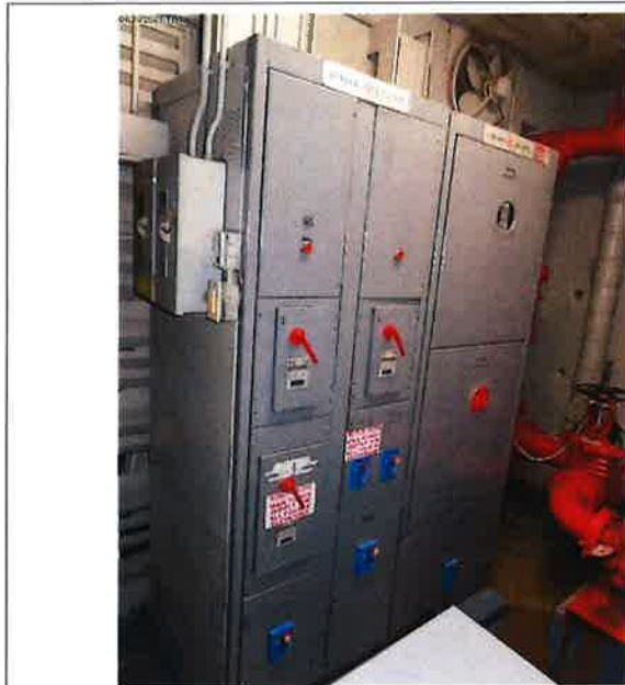
Photo # 1. Unidentified service-disconnect switch (main electrical room North building)
