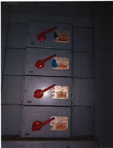
Photo # 27. North building - electrical panel depicted (item #4.13)
