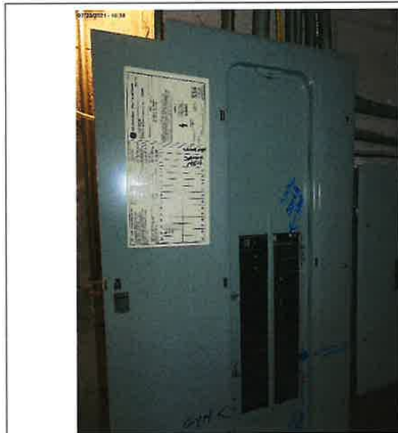
Photo # 39. North building - electrical panel depicted (item #4.25)
