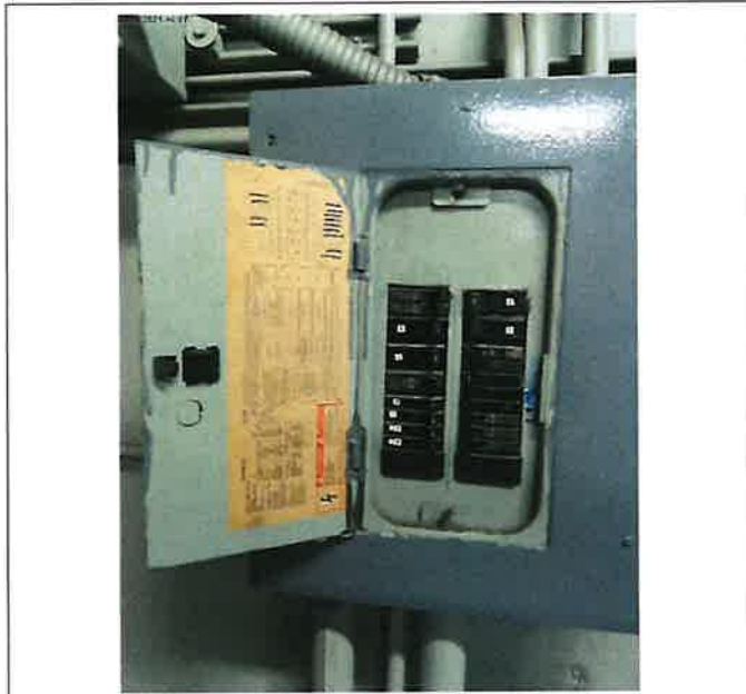
Photo # 53. South building main electrical room electrical panel depicted (item #4.38)
