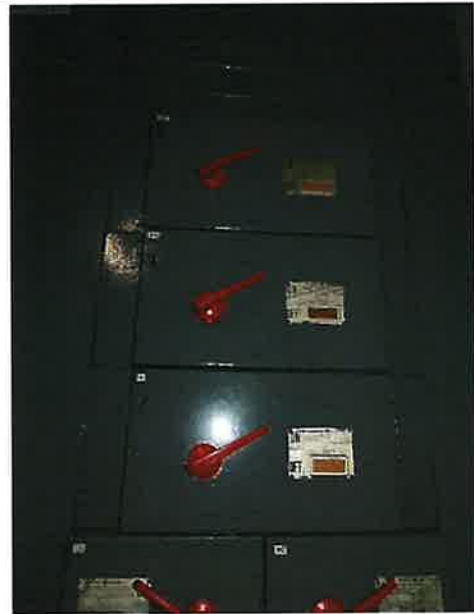
Photo # 20. North building main electrical room electrical panel depicted (item #4.6)
