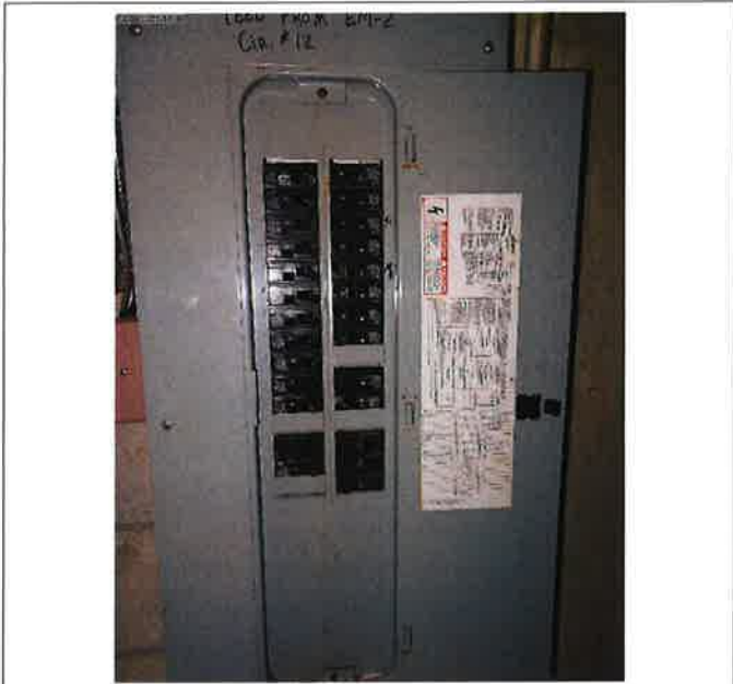
Photo # 81. South building - electrical panel depicted (item #4.64)
