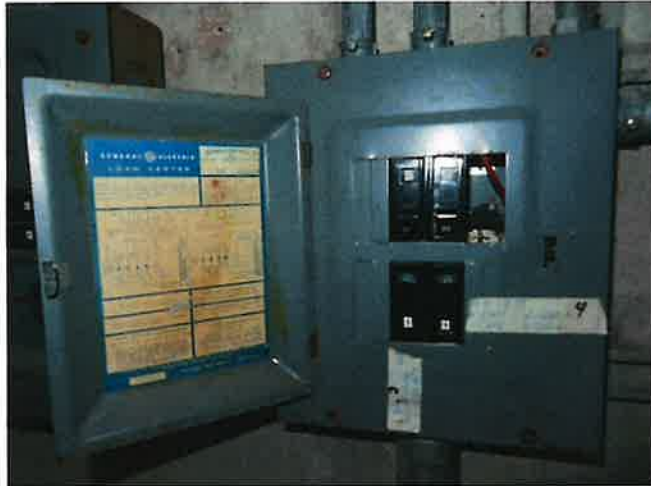
Photo # 79. South building - electrical panel depicted (item #4.62)
