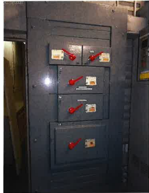
Photo # 22. North building main electrical room electrical panel depicted (item #4.8)
