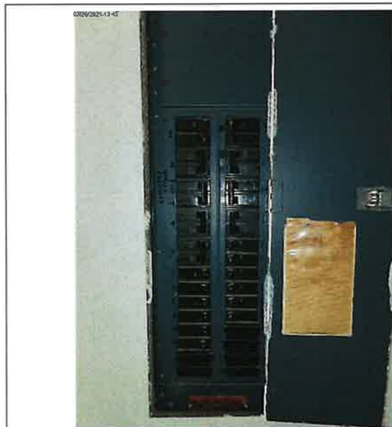
Photo # 71. South building - electrical panel depicted (item #4.57)
