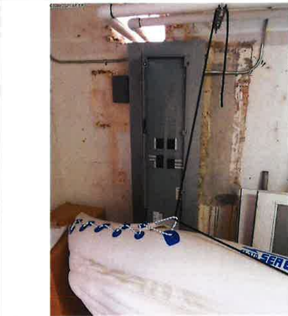
Photo # 87. Marina storage room (under the pool deck) – electrical panel depicted (item #4.70)
