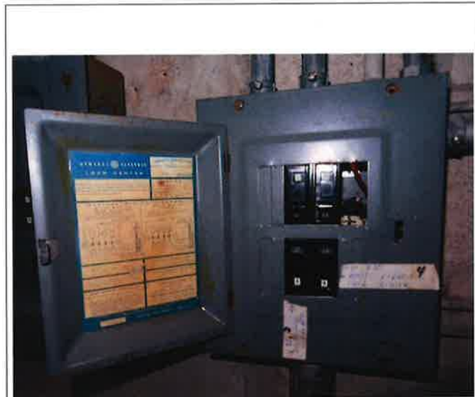
Photo # 79. South building - electrical panel depicted (item #4.62)
