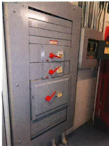
Photo # 58. South building main electrical room electrical panel depicted (item #4.43)
