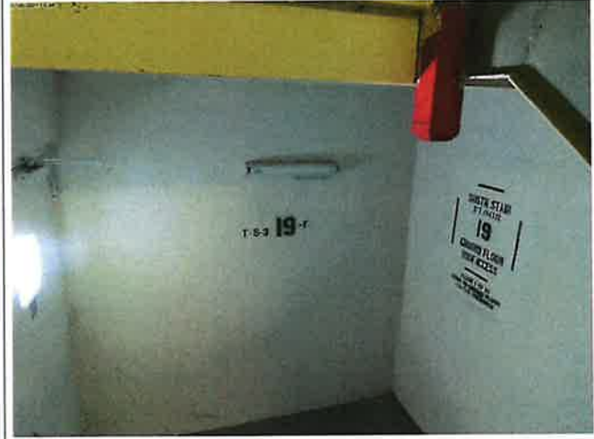
Photo # 136. Insufficient illumination for the building means of egress (Item #13.SOUTH-b).
