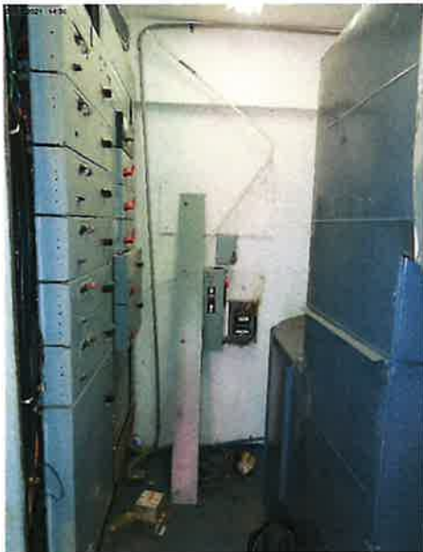
Photo # 127. Working space clearance violation (Item # 10-SOUTH-h)
