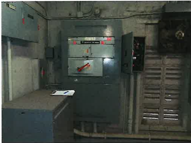
Photo # 3. Unidentified service-disconnect switch (main electrical room South building)
