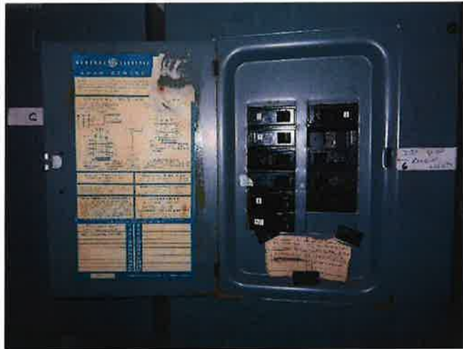
Photo # 49. North building - electrical panel depicted (item #4.35)
