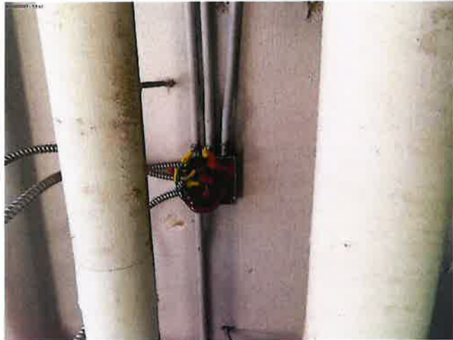
Photo # 109. Opening in junction boxes/enclosures (Item #10.f.2)
