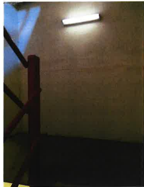
Photo # 138. Insufficient illumination for the building means of egress (Item #13.SOUTH-c).
