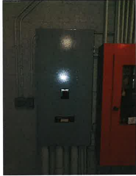
Photo # 2. Unidentified service-disconnect switch (main electrical room South building)
