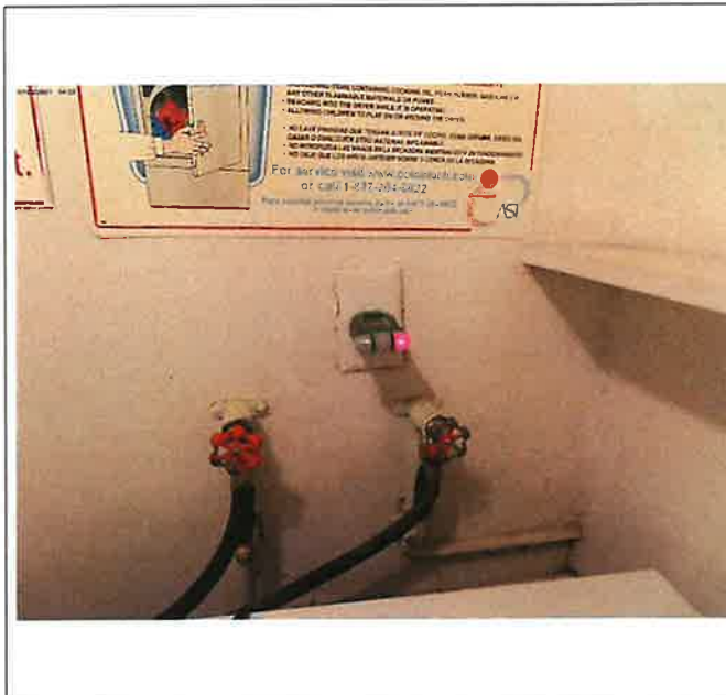
Photo # 97. Laundry room receptacle for the washer machine is depicted. Notice the grounding is missing. Also, GFCI protection is required (typical for all level, all towers in both buildings) (Item #10.b)
