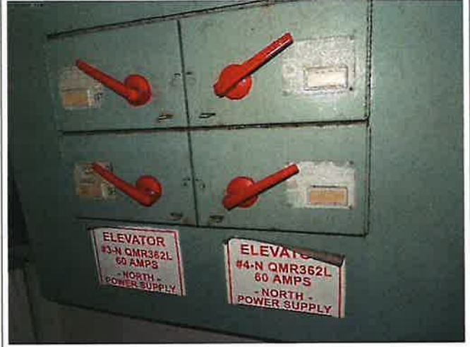
Photo # 26. North building - electrical panel depicted (item #4.12)
