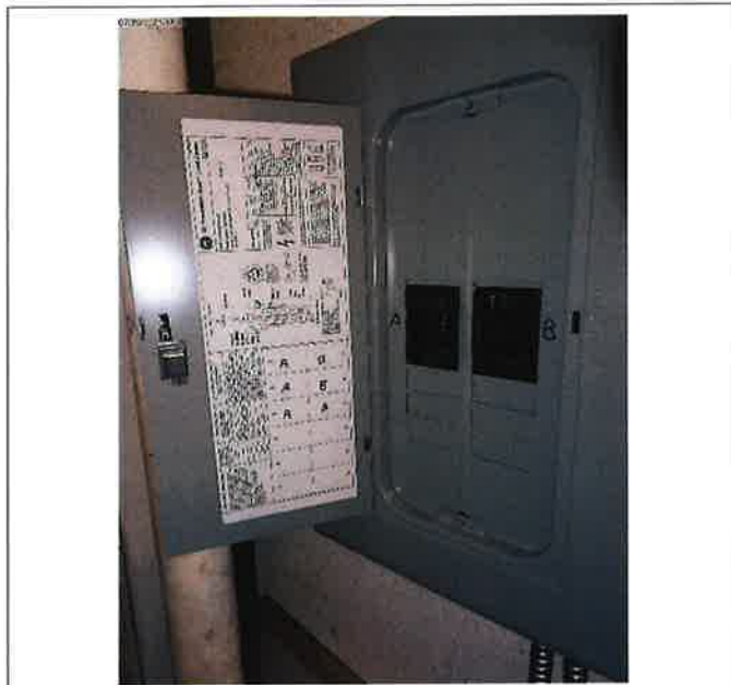
Photo # 77. South building - electrical panel depicted (item #4.60)
