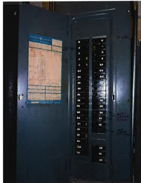
Photo # 46. North building - electrical panel depicted (item #4.32)
