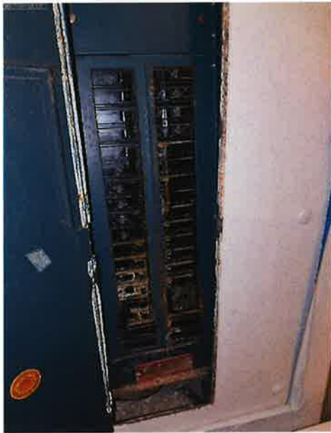
Photo # 75. South building - electrical panel depicted (item #4.59)
