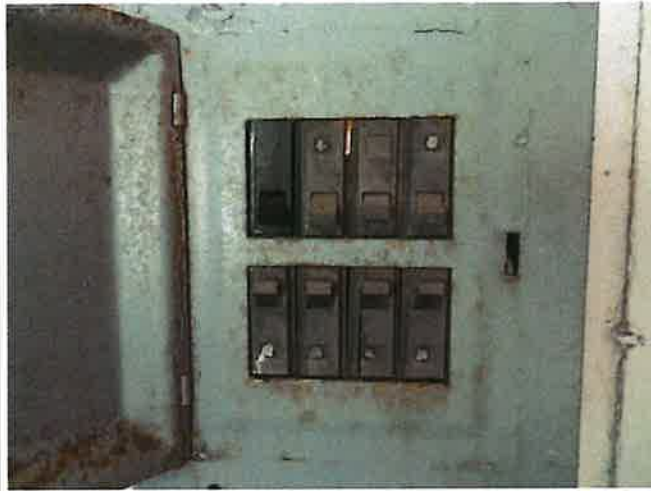
Photo # 25. North building - electrical panel depicted (item #4.11)
