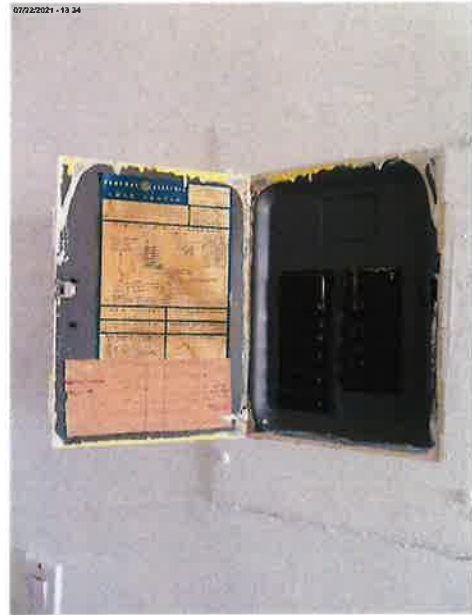
Photo # 90. Typical residential panel where the circuit directory is missing, incomplete or confusing (item #4.71)
