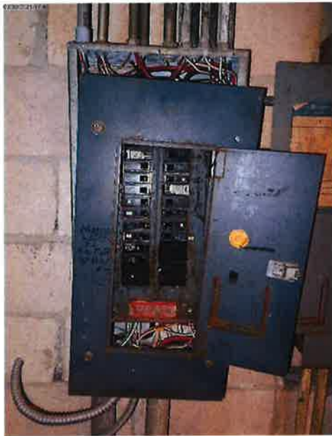
Photo # 43. North building - electrical panel depicted (item #4.29)
