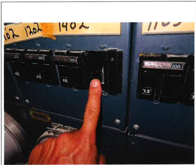
Photo # 11. South building, tower 3, meter room level 12: opening in circuit breaker space.
