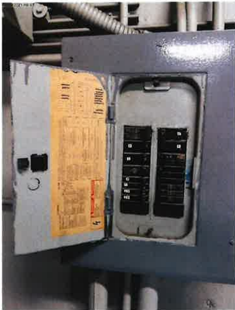
Photo # 53. South building main electrical room electrical panel depicted (item #4.38)
