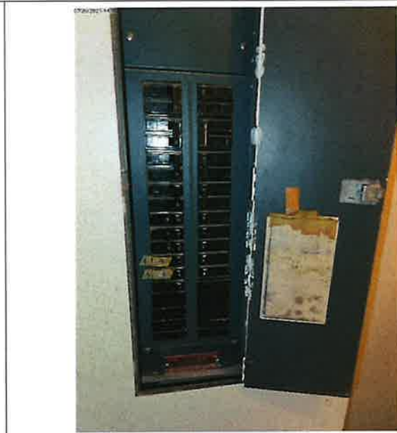
Photo # 70. South building - electrical panel depicted (item #4.55)
