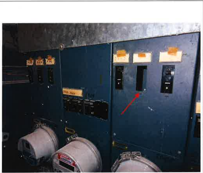
Photo # 10. South building, tower 4, meter room level 19: opening in circuit breaker space.
