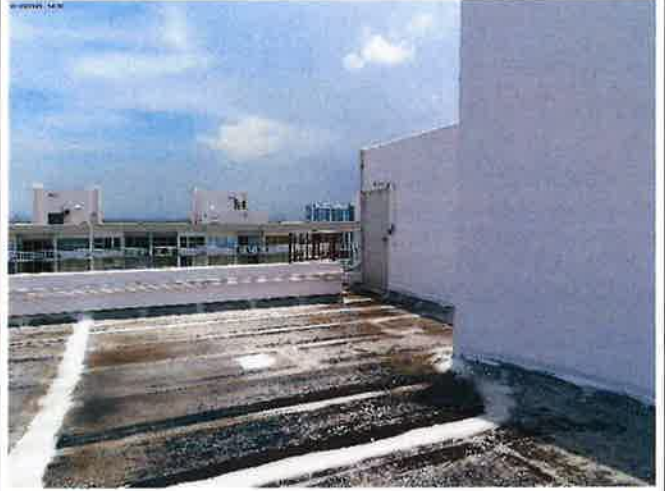
Photo # 142. North building roof: Stairwell exit doors are missing exit sign (Item # 16.a)
