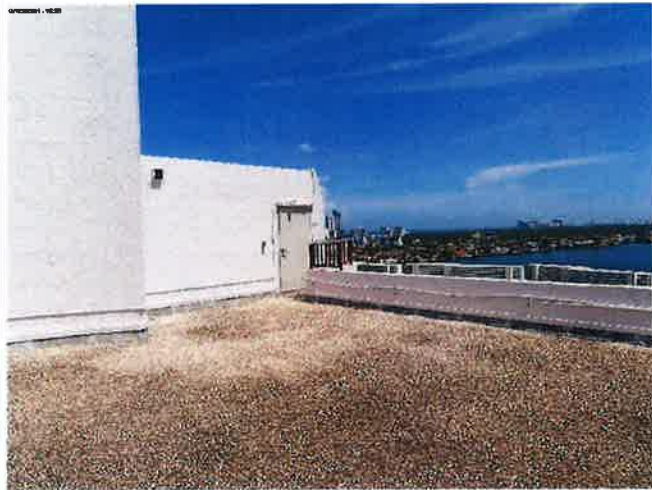
Photo # 147. South building roof: Stairwell exit doors are missing exit sign (Item # 16.b)
