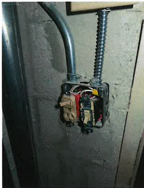
Photo # 119. Receptacle and switch without cover (Item # 10-SOUTH-d)
