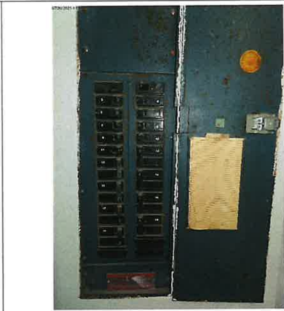
Photo # 38. North building - electrical panel depicted (item #4.24)
