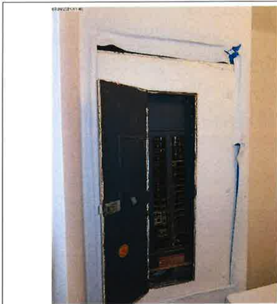
Photo # 73. South building - electrical panel depicted (item #4.59)
