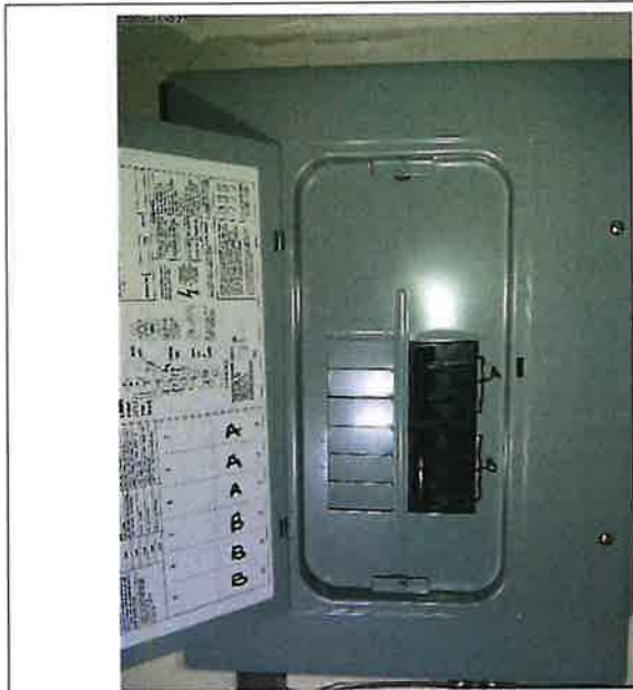
Photo # 45. North building - electrical panel depicted (item #4.31)
