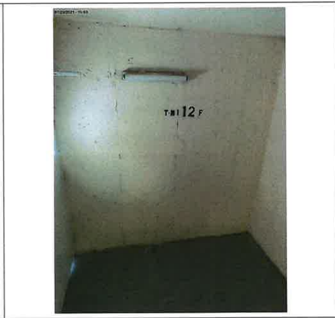
Photo # 132. Insufficient illumination for the building means of egress (Item #13.NORTH-d).
