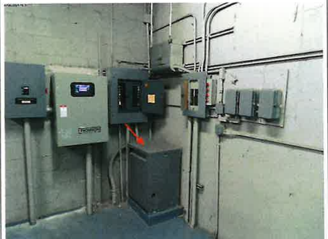
Photo # 52. South building main electrical room electrical panel depicted (item #4.37)
