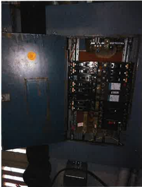
Photo # 17. North building main electrical room electrical panel depicted (item #4.3)
