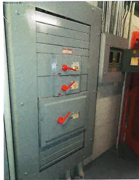
Photo # 58. South building main electrical room electrical panel depicted (item #4.43)
