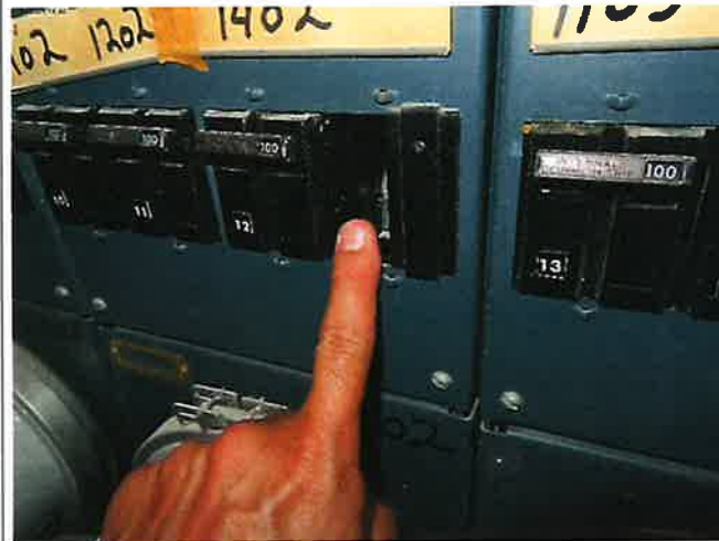
Photo # 11. South building, tower 3, meter room level 12: opening in circuit breaker space.
