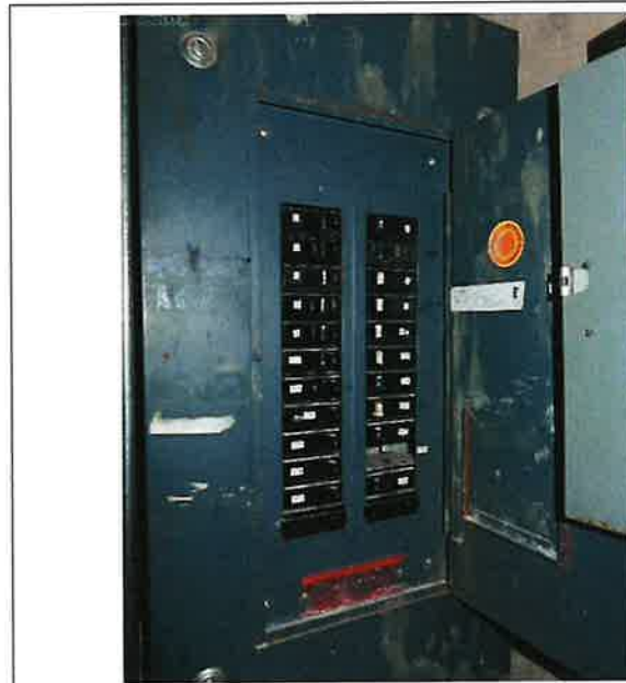
Photo # 47. North building - electrical panel depicted (item #4.33)
