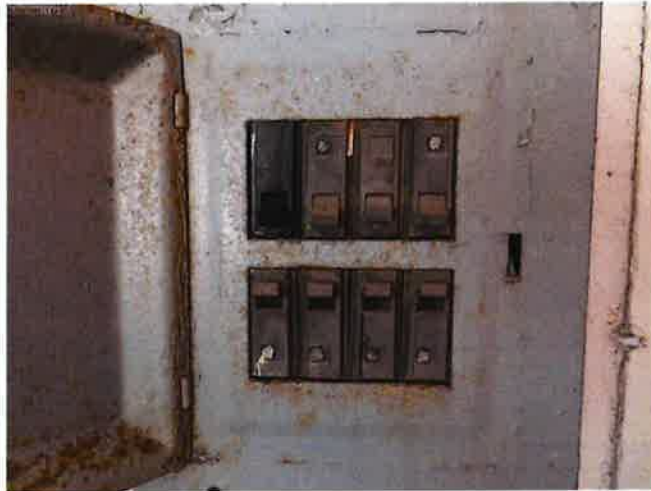
Photo # 25. North building - electrical panel depicted (item #4.11)
