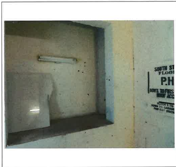
Photo # 129. Insufficient illumination for the building means of egress (Item #13.NORTH-a).
