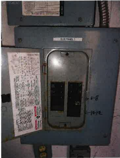
Photo # 29. North building - electrical panel depicted (item #4.15)
