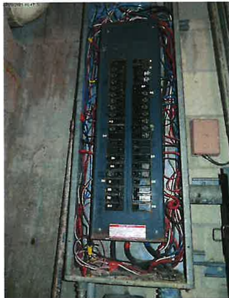
Photo # 83. South building - electrical panel depicted (item #4.66)
