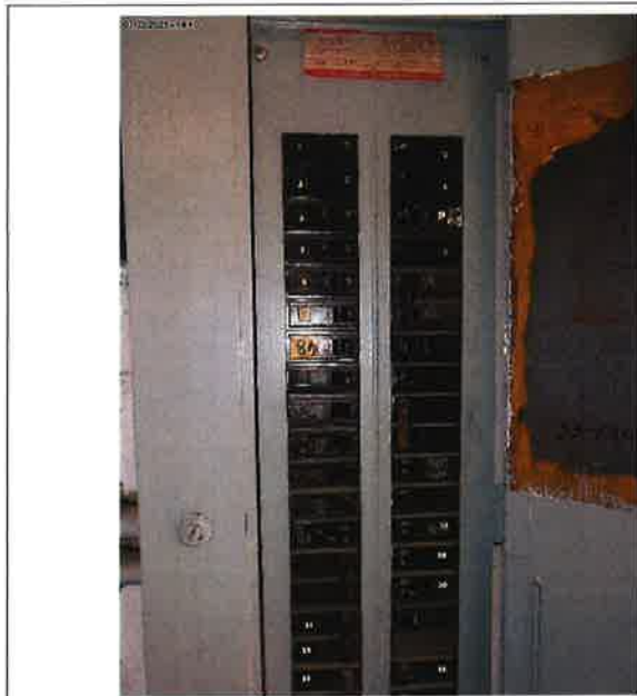
Photo # 61. South building - electrical panel depicted (item #4.48)
