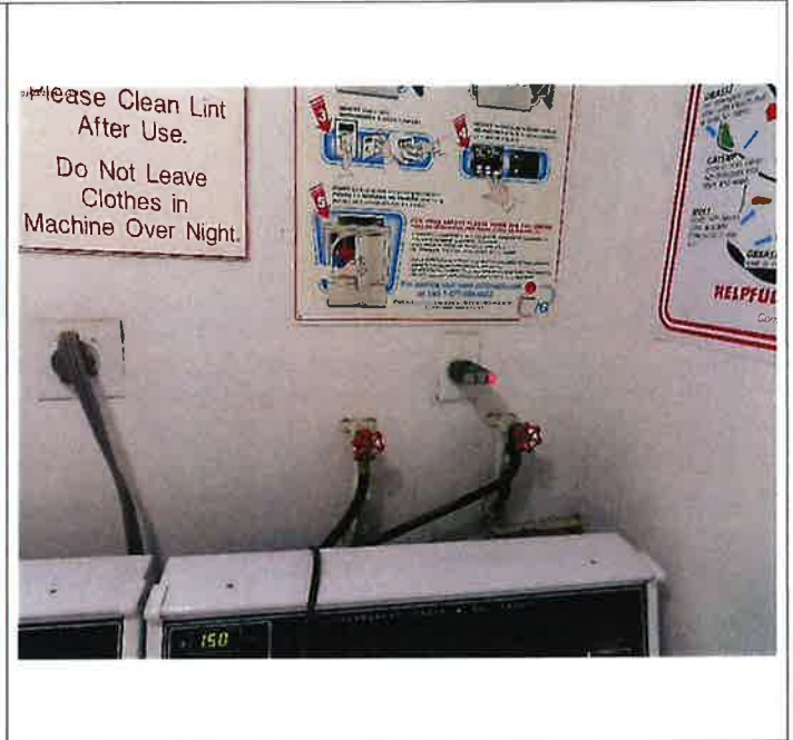
Photo # 98. Laundry room receptacle for the washer machine is depicted. Notice the grounding is missing. Also, GFCI protection is required (typical for all level, all towers in both buildings) (Item #10.b)
