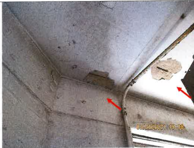
South Roof AHU4
