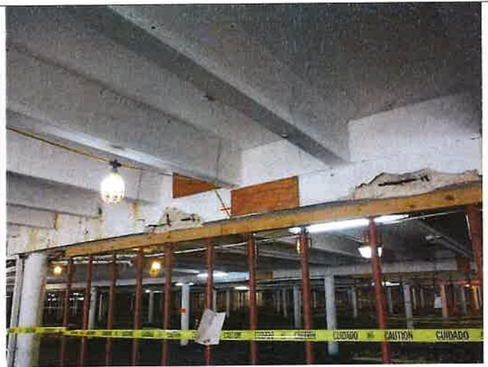
Picture 32 Plaza Del Prado West Deck and Garage observed with concrete spalling and exposed corroded rebar.
