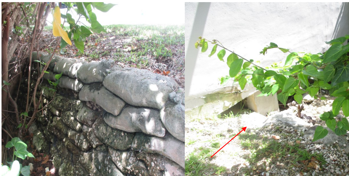
Image 7: Photo on right, preformed concrete riprap retaining wall and left damage section.
